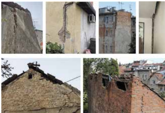
Figure 19. Detachment of gable wall and typical cracks in internal part of the building (photos courtesy of Mario Todorčić and [39])
