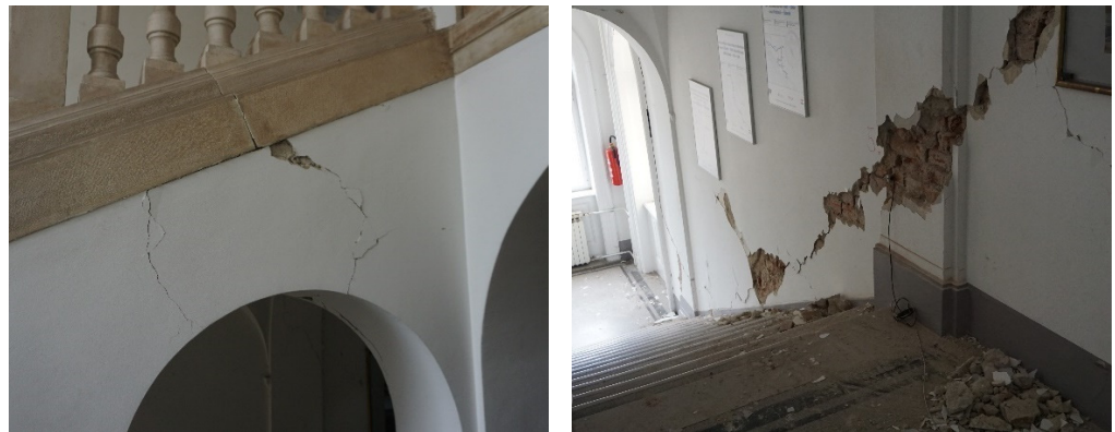
Figure 4. Damage to the central staircase in the HŽI head-office building.
