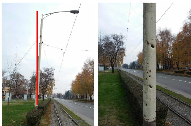
Fig. 2. Example of substantially damaged columns.
