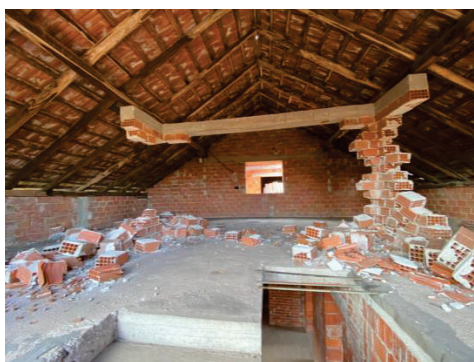
Figure 12: Improper attic modifications (photo credit: HCPI [4])
