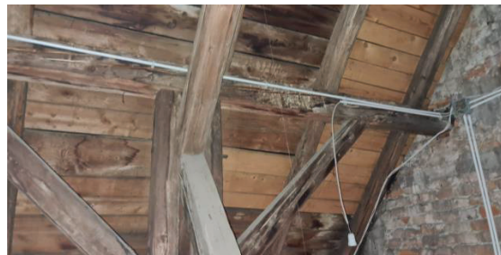
Figure 9: Failure of timber elements due to water leakage and seismic excitations (photo credit: Studio Arhing d.o.o.)
