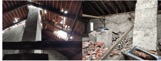
Figure 8: Failure of chimneys (from inside) (photo credit: M. Stepinac)
