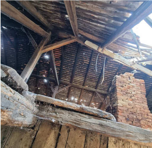
Figure 5: Failure of timber elements due to chimney failure (photo credit: R. Gulić)
