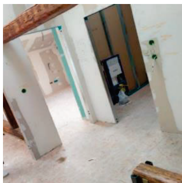
Figure 11: Improper attic modifications (photo credit: HCPI [4])
