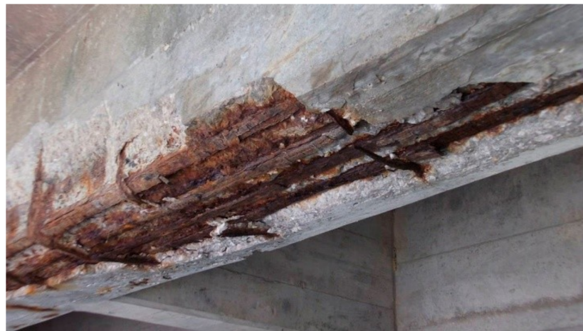
Figure 2. Display of reinforcement corrosion effects in reinforced concrete beam.
