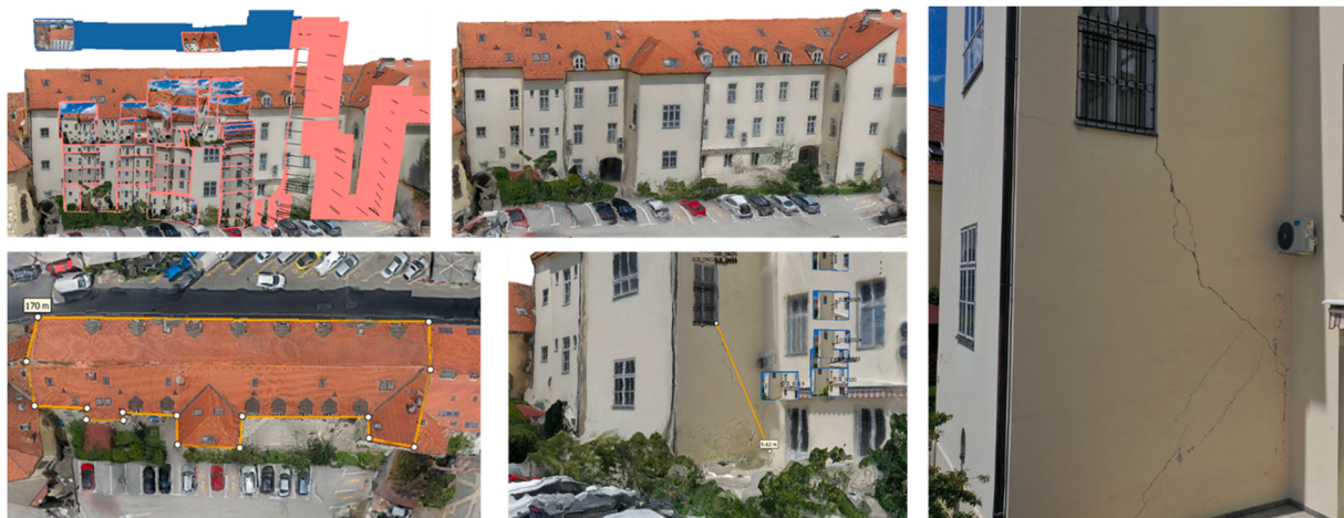
Fig. 9. Photogrammetric view of the building, respectively with positions of the camera, photogrammetric model, measuring of the roof geometry, measuring of a crack, photo of a crack.
