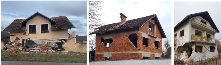
Fig. 19 Damage to URM family houses including a collapse due to irregularity in elevation (left) and combined in-plane and out-of plane failures due to lack of vertical confinement (centre and right) (CCEE 2022)
