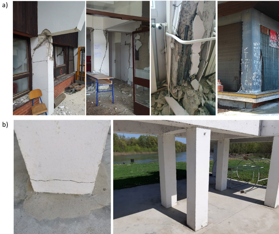
Fig. 24 Typical damage to RC building: a brittle fractures and b bending cracks in columns (CCEE 2022)
