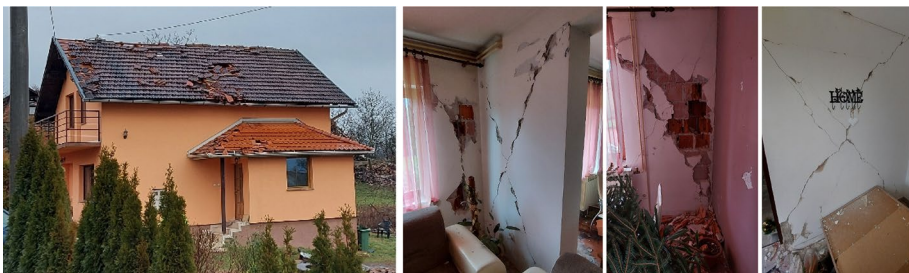
Fig. 21 Damage to confined masonry family houses (CCEE 2022)
