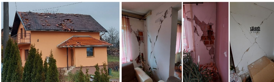
Fig. 21 Damage to confined masonry family houses (CCEE 2022)
