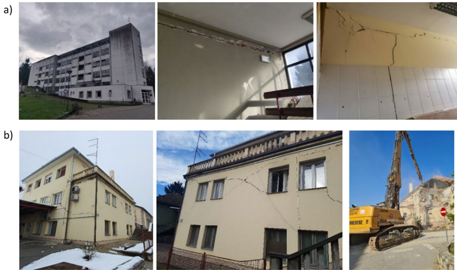
Fig. 10 Petrinja, damage to buildings in the health sector: a Special hospital for chronic diseases and b Health center in Petrinja (photos: private collection of authors and courtesy of Tina Nikolić, Joning d.o.o.)
