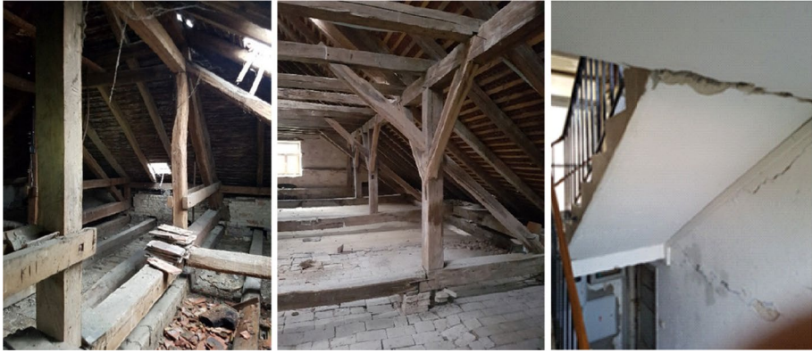
Fig. 22 Damage to roof structures and staircases (CCEE 2022)
