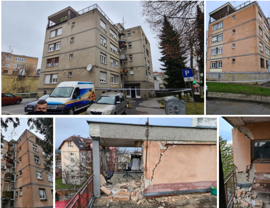
Fig. 23 Damage to multi-storey residential buildings in Zaprešić, located more than 60 km from the epicenter (CCEE 2022)
