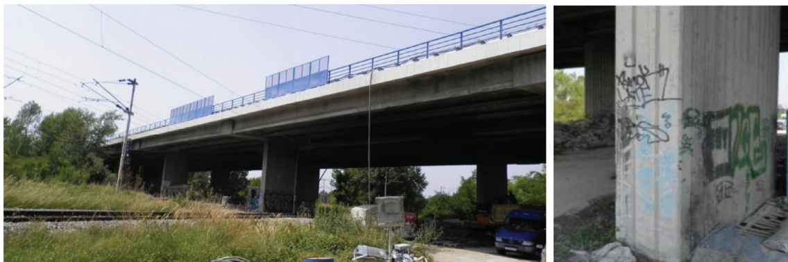
Fig. 1: View of Klara jug bridge (left); column used for experimental work (right).
