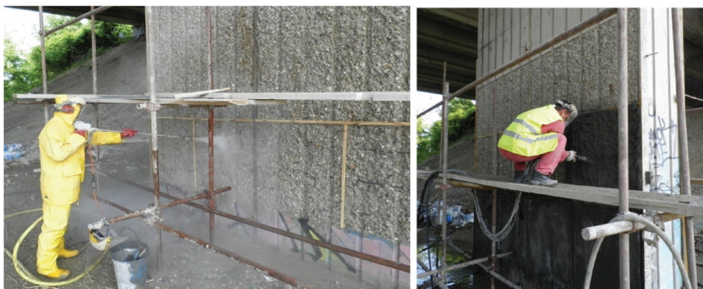
Fig. 2: Surface preparation by hydrodemolition under high pressure to a depth of 1.5 cm, (left) and spraying of repair mortar (right).
