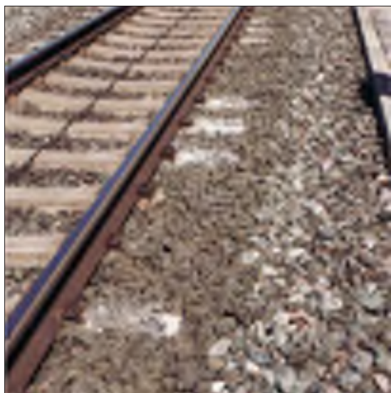
Figure 1 White spots; Rapid ballast degradation along a bridge deck
