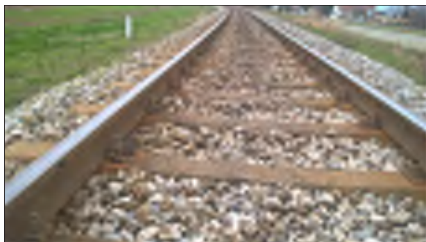
Figure 5 Condition of track type 4
