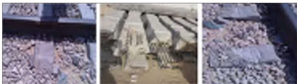
Figure 1 Cracked and Corroded Concrete Sleepers (km 19, 25, 31 & 37)
