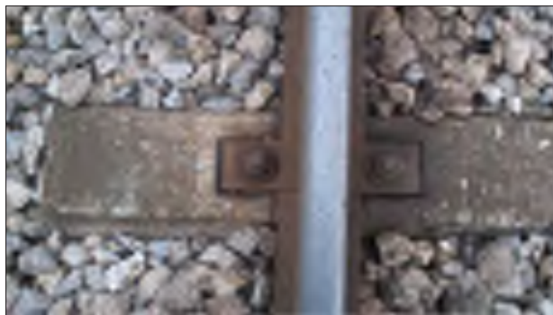
Figure 3 Condition of track type 3
