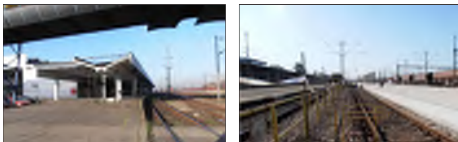
Figure 3 Railway stations Slavonski Brod and Vinkovci in the initial phases of reconstruction
