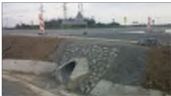
Figure 8 Completed culvert at roundabout entrance (first phase of construction) during construction work
