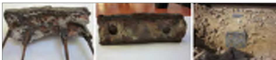
Figure 2 Severe corrosion on anchor plate & rebar, on anchor plate
