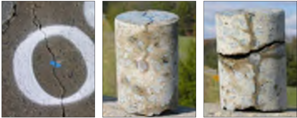
Figure 1 Vertical crack on the surface of a bridge deck (left), a core with a vertical crack (middle), and a core with a vertical crack and delamination (right)
