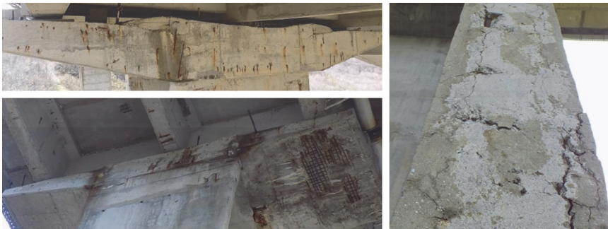
Figure 11. Deterioration of reinforced concrete due to corrosion at Bukovo Viaduct in Croatia
