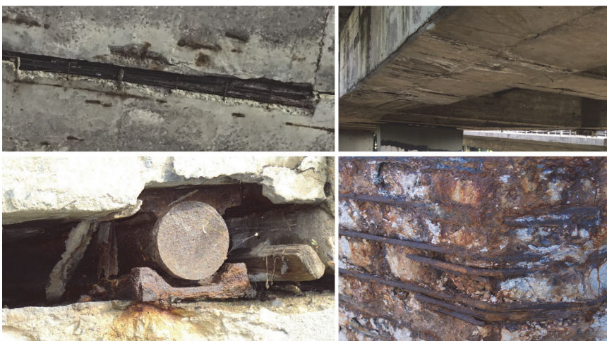
Figure 12. Deterioration of reinforced concrete due to corrosion at bridges in Zagreb, Croatia
