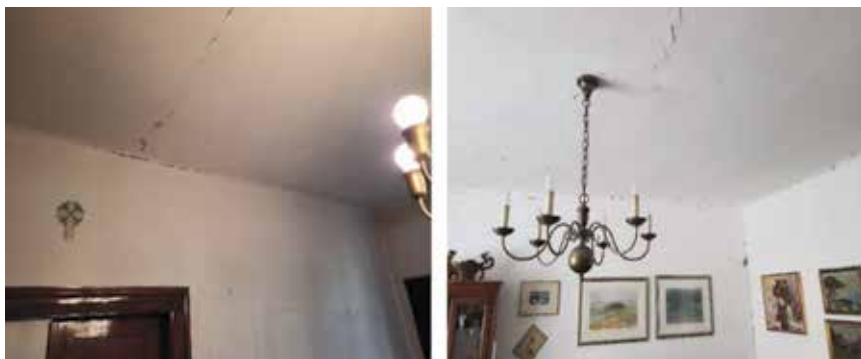
Figure 24. Cracks at ceilings [39]
