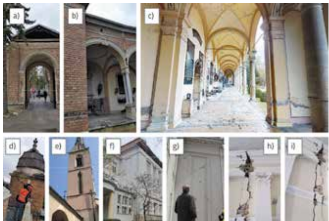
Figure 30. Earthquake damage to some notable buildings: Mirogoj Cemetery (a.-d.), Franciscan Monastery at Kaptol (e), registry office building of the Faculty of Medicine at Šalata (f.-g.), University and Faculty of Law building (h.-i.) [39]
