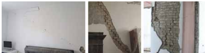
Figure 22. Diagonal cracks in load bearing walls [39]
