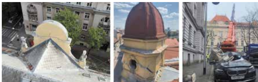
Figure 21. Damage of decorative elements (photos courtesy of Mario Todorčić and [39])
