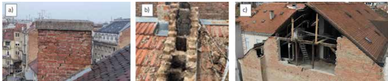
Figure 17. Collapse of chimneys and top part of the gable walls (photo courtesy of Mario Todorčić and [39])
