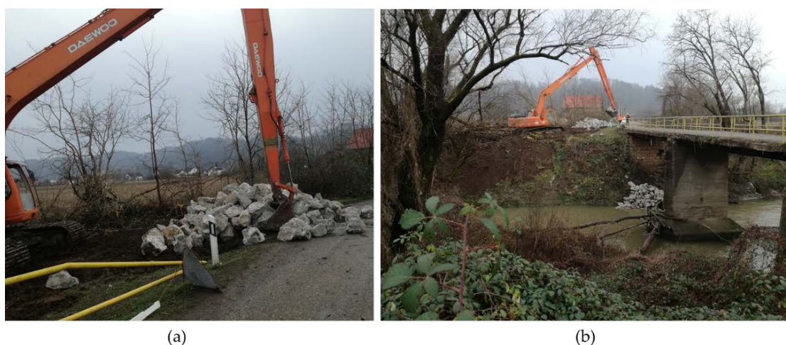
Figure 15. (a) Stone material for urgent stabilization; (b) placing of the additional weight on the abutment and embankment.
