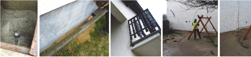
Figure 7. Three photos from Petrinja: a manhole filled with sand due to liquefaction, ejecta on the other side of the house and the consequent cracking; cracks around the balcony due to settlement caused by liquefaction across the street. Two photos from Brest Pokupski: a cracked house and thick layer of ejecta after liquefaction – the crack spread through several yards and filled several houses with up to 50 cm of sand
