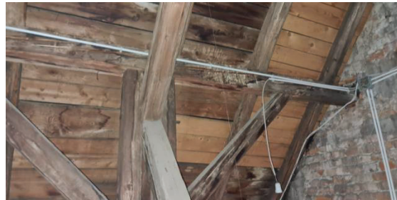
Figure 9: Failure of timber elements due to water leakage and seismic excitations (photo credit: Studio Arhing d.o.o.)
