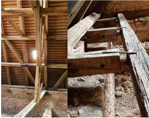
Figure 10: Bad detailing (photo credit: Studio Arhing d.o.o.)
