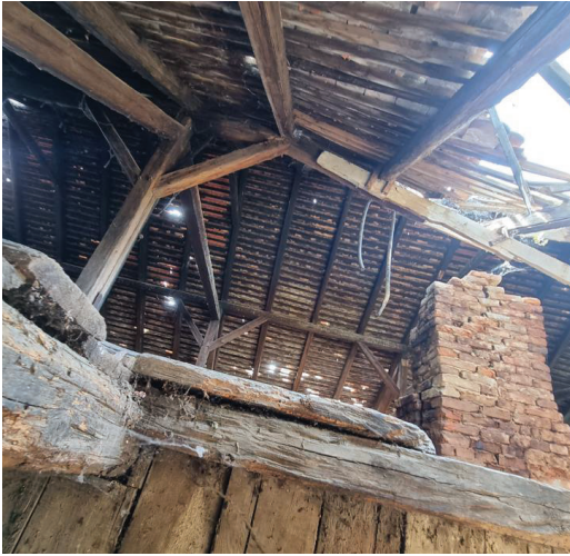
Figure 5: Failure of timber elements due to chimney failure (photo credit: R. Gulić)
