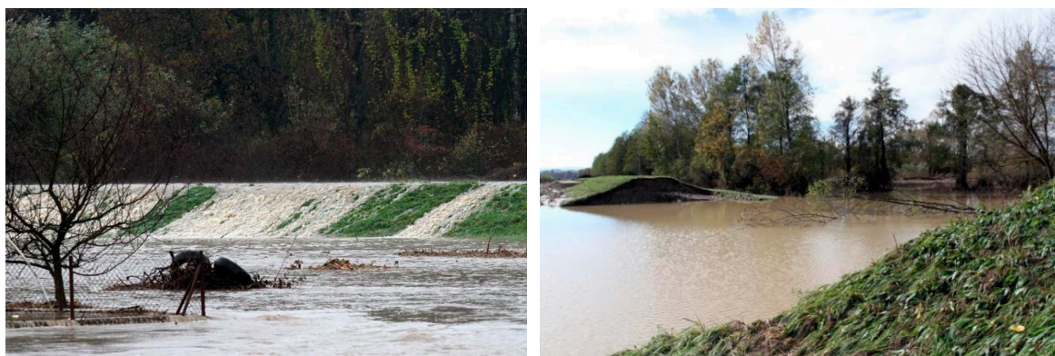
Figure 1. Overtopping and breach in Otok Virje-Brezje levee [34].
