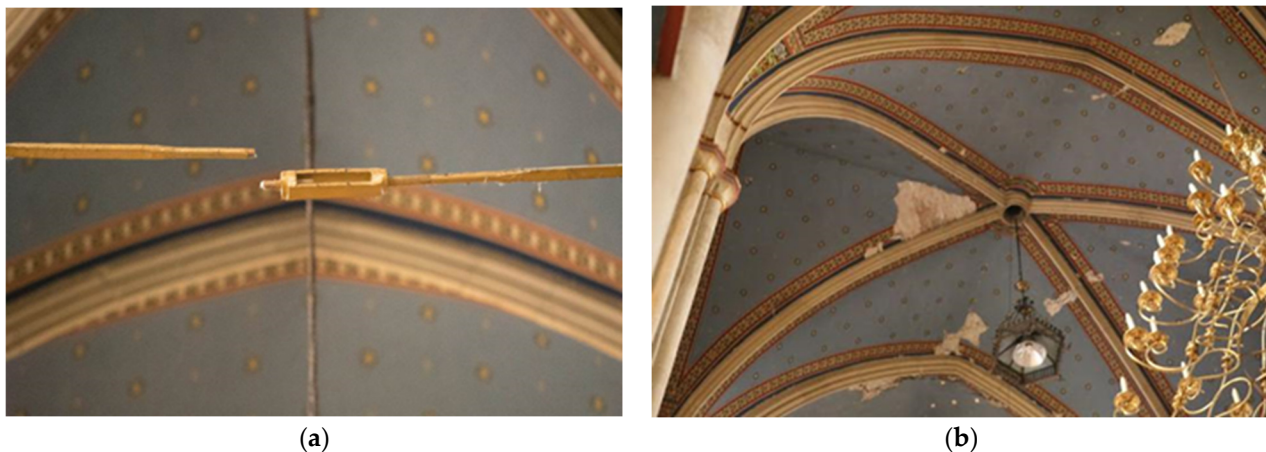
Figure 1. Cathedral of the Assumption of Mary, Zagreb: (a) Fractured tie rod after its load bearing capacity was reached (b) Damaged vaults after the March 22nd 2020 Zagreb earthquake.
