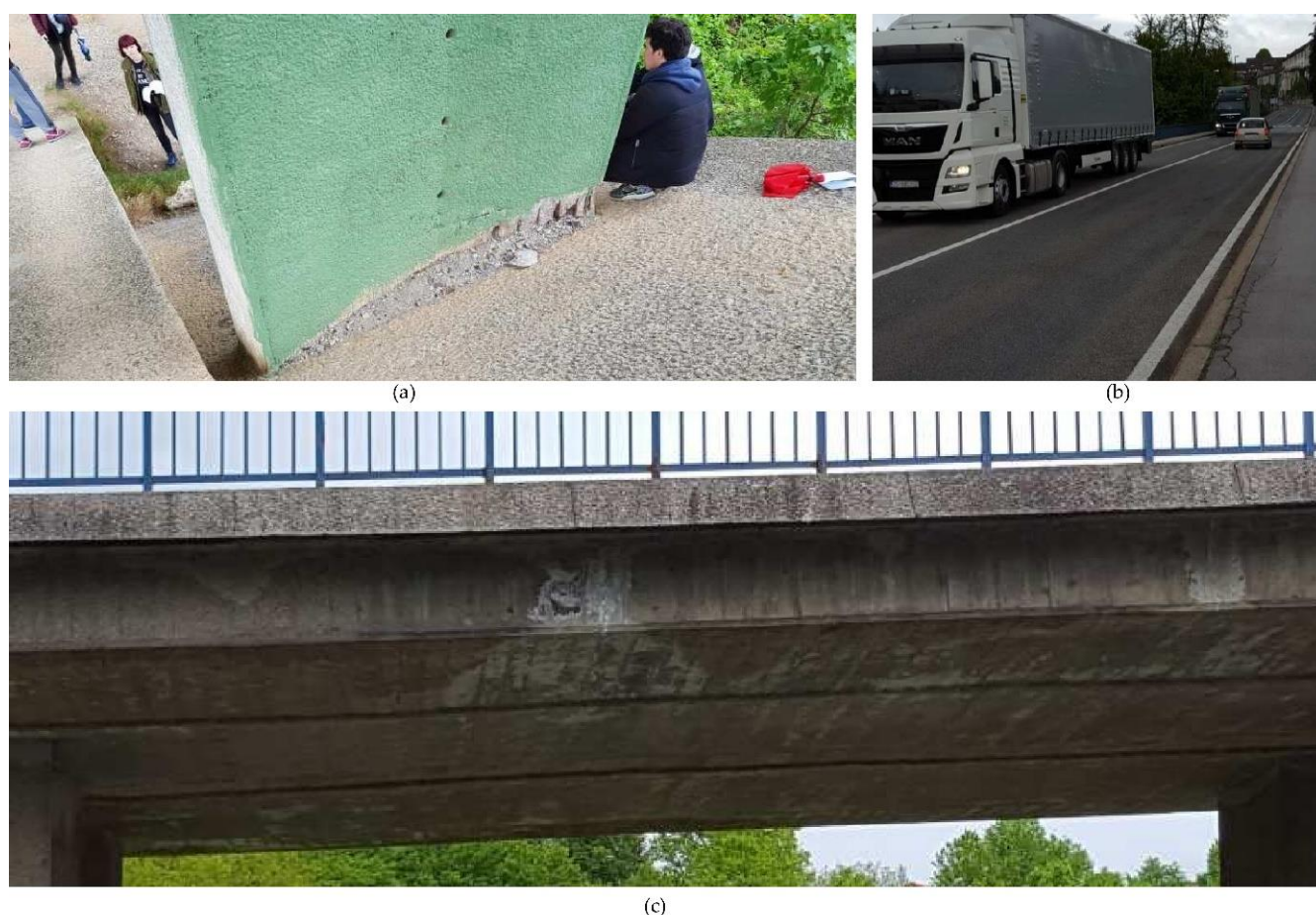
Figure 4. Most significant damages to Slunjčica Bridge [48]: (a) concrete cover fraction and reinforcing steel corrosion at the pier due to the insufficient concrete cover and poor construction; (b) sidewalk block cracking probably due to vibration and poor construction concrete; (c) cover fraction and reinforcing steel corrosion at the slab bottom due to insufficient concrete cover and efflorescence appearance due to wetting and probable damage in waterproofing. Reprinted with permission from ref. [48]. 2019. IABSE.
