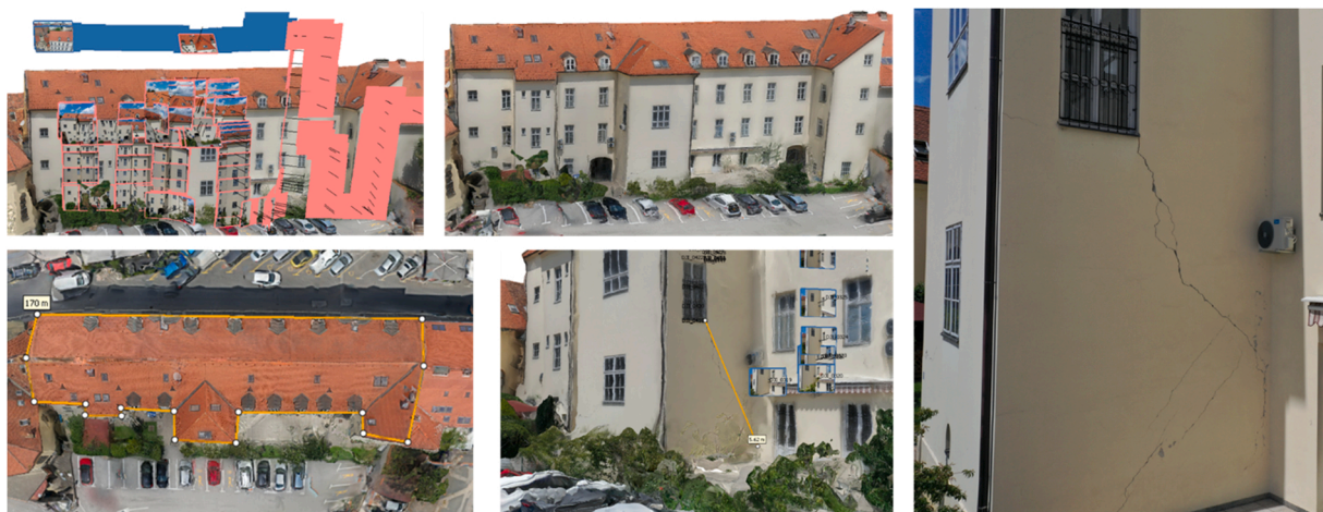
Fig. 9. Photogrammetric view of the building, respectively with positions of the camera, photogrammetric model, measuring of the roof geometry, measuring of a crack, photo of a crack.
