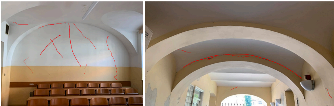
Fig. 6. Characteristic cracks, marked with a red line (photo credit: Mislav Stepinac).
