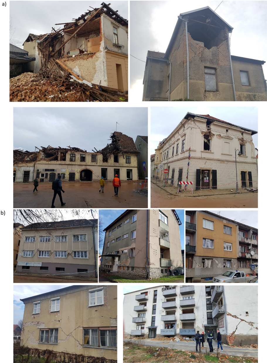
Fig. 17 Damage to unreinforced masonry buildings: a out-of-plane failure mechanisms, b in-plane failure mechanisms (CCEE 2022)
