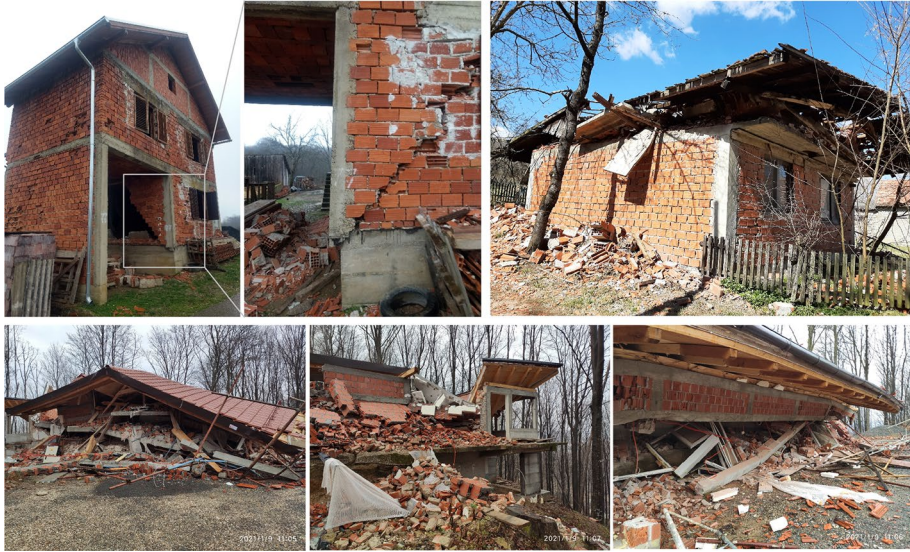
Fig. 20 Damage to (partially) confined masonry with significant structural deficiencies family houses (CCEE 2022)
