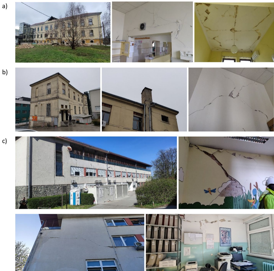
Fig. 9 Sisak, damage to buildings in the health sector, Hospital "Dr. Ivo Pedišić": a Internal clinic, b Administrative building, and c Pediatrics building (CCEE 2022)
