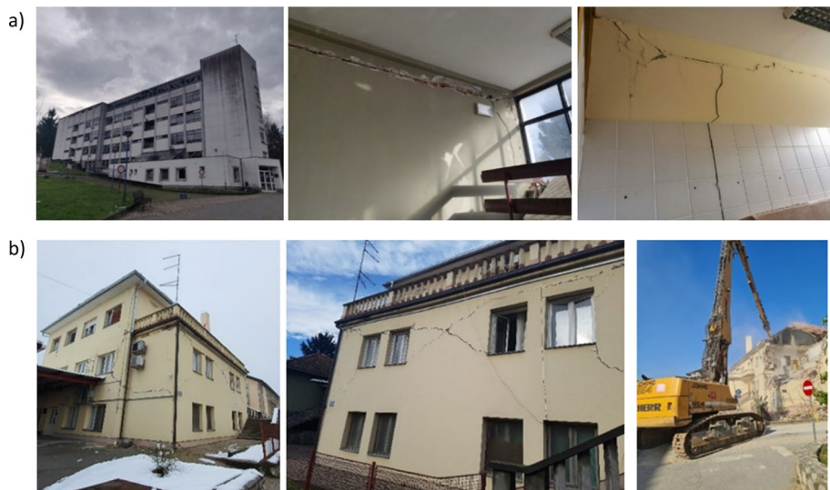
Fig. 10 Petrinja, damage to buildings in the health sector: a Special hospital for chronic diseases and b Health center in Petrinja (photos: private collection of authors and courtesy of Tina Nikolić, Joning d.o.o.)
