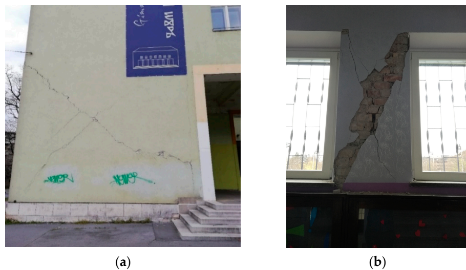
Figure 3. Observed characteristic damages on (a) the load bearing walls (b) the walls between the openings.
