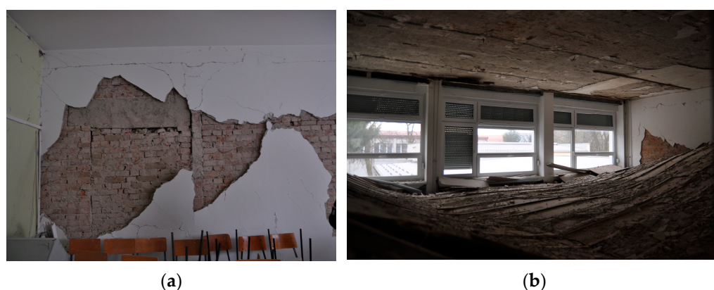
Figure 4. Observed damage on (a) the partition wall and (b) the ceiling.
