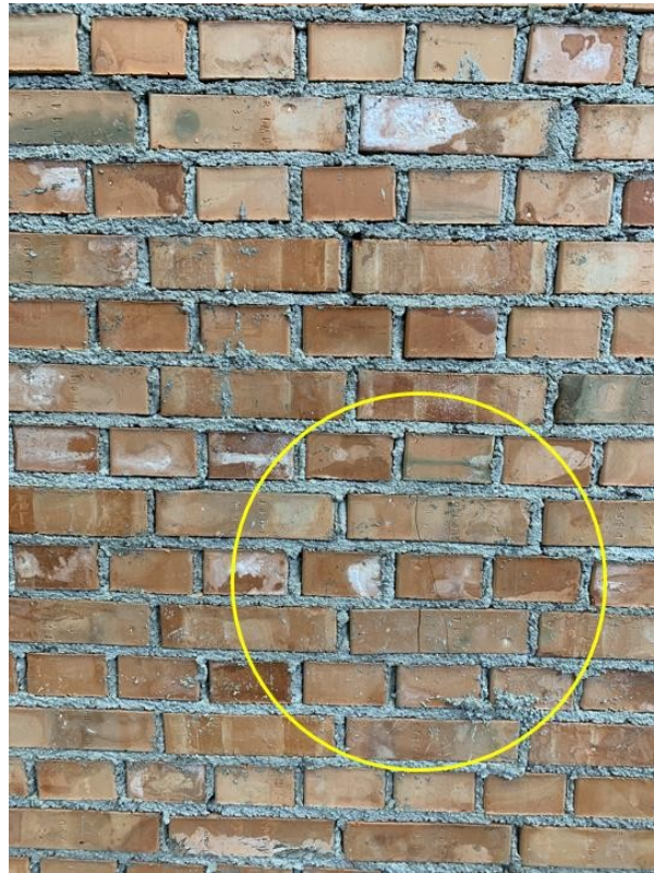
Figure 4.32 First crack of URM 3 pier
