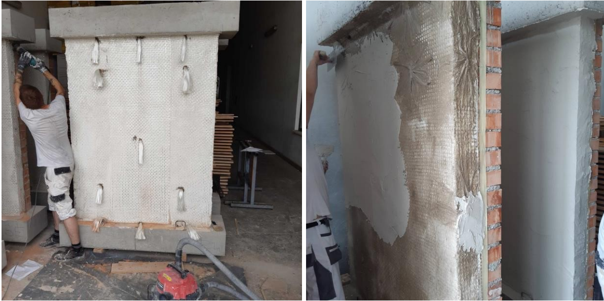
Figure 4.6 Installation of transversal connectors and application of the final layer of the mortar matrix
