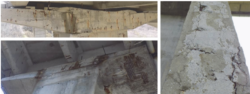
Figure 11. Deterioration of reinforced concrete due to corrosion at Bukovo Viaduct in Croatia
