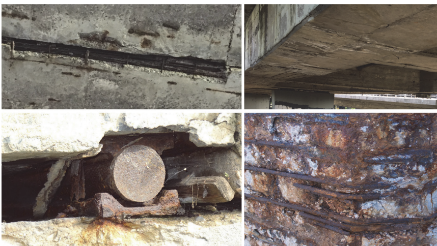
Figure 12. Deterioration of reinforced concrete due to corrosion at bridges in Zagreb, Croatia
