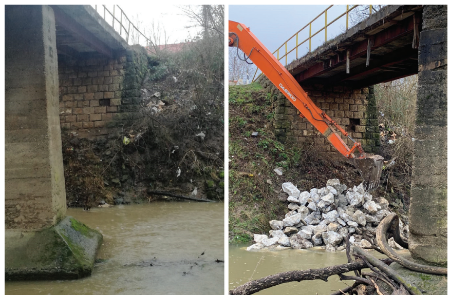
Figure 8. Damage to bridge substructure after earthquake in Petrinja (left) and temporary retrofitting in order to open the bridge to traffic (right)
