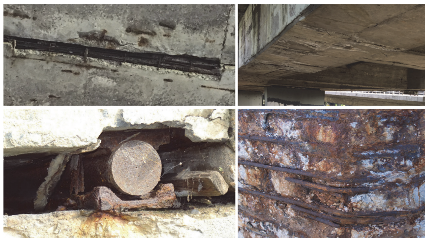
Figure 12. Deterioration of reinforced concrete due to corrosion at bridges in Zagreb, Croatia
