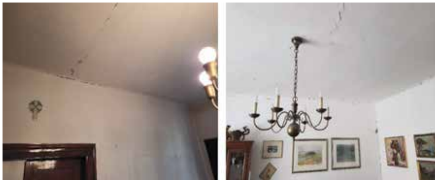
Figure 24. Cracks at ceilings [39]
