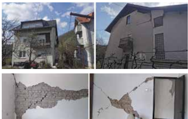
Figure 29. Damage to houses at LB Dankovec, CD Gornja Dubrava (photo courtesy of Luka Božić and [39])
