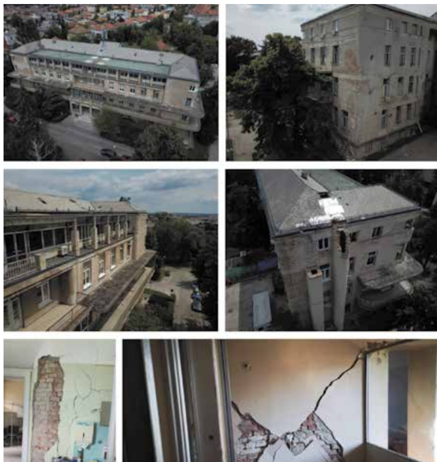
Figure 37. View of damage to building of Orthopaedics Clinic
