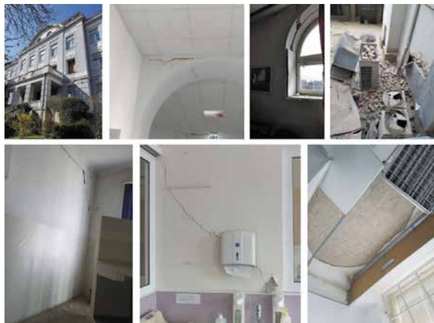
Figure 36. Damage to the Old building of Clinic for Women’s Health and Obstetrics in Petrova
