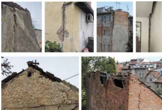
Figure 19. Detachment of gable wall and typical cracks in internal part of the building (photos courtesy of Mario Todorčić and [39])
