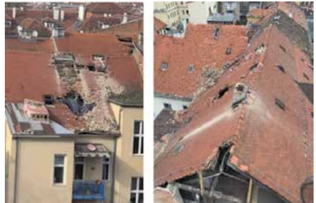
Figure 20. Roof structure damage (photos courtesy of Mario Todorčić)
