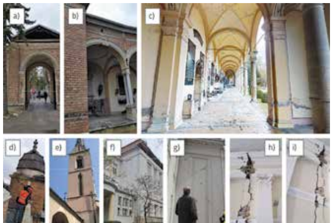
Figure 30. Earthquake damage to some notable buildings: Mirogoj Cemetery (a.-d.), Franciscan Monastery at Kaptol (e), registry office building of the Faculty of Medicine at Šalata (f.-g.), University and Faculty of Law building (h.-i.) [39]
