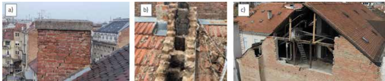
Figure 17. Collapse of chimneys and top part of the gable walls (photo courtesy of Mario Todorčić and [39])
