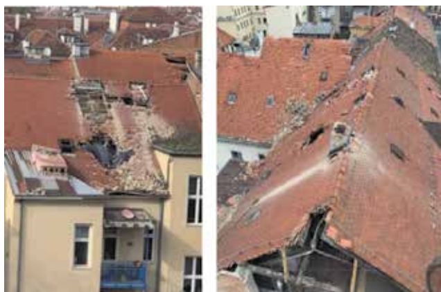
Figure 20. Roof structure damage (photos courtesy of Mario Todorčić)
