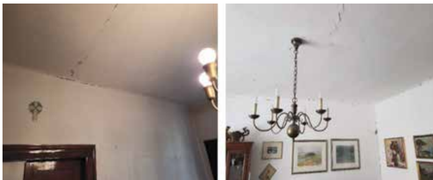
Figure 24. Cracks at ceilings [39]
