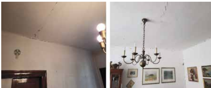
Figure 24. Cracks at ceilings [39]
