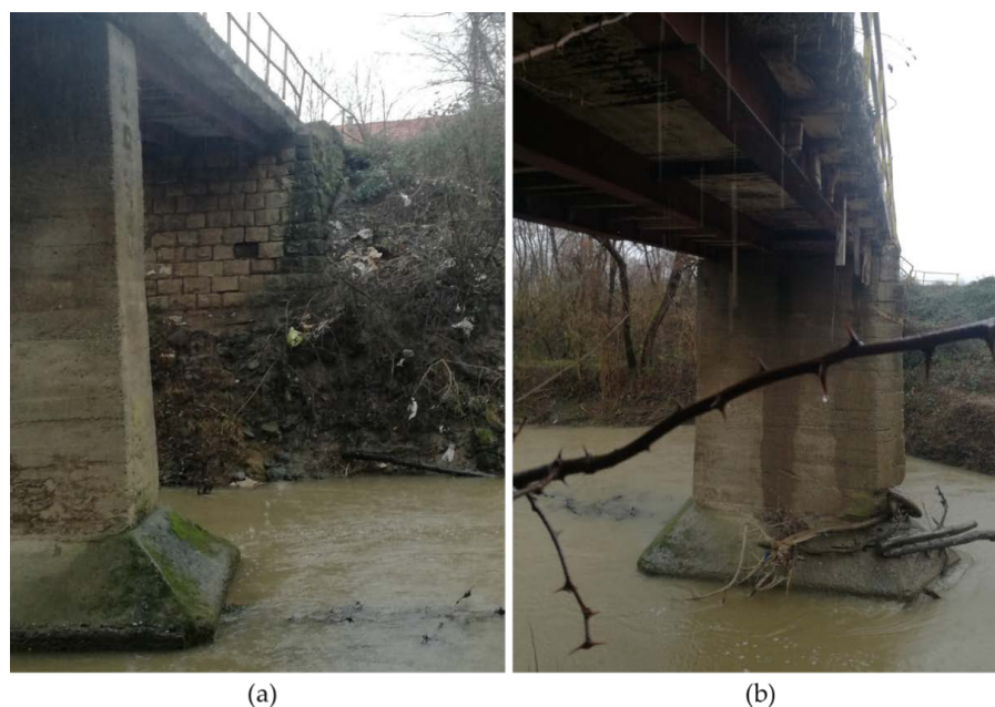
Figure 13. (a) Masonry abutment and (b) composite superstructure of the bridge to Majske Poljane.
