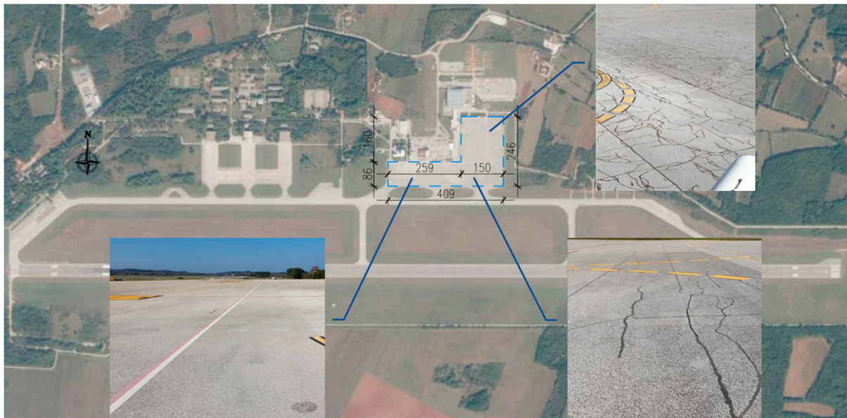
Figure 1. Pula Airport apron with pavement distresses.
