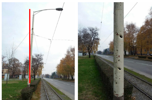
Fig. 2. Example of substantially damaged columns.
