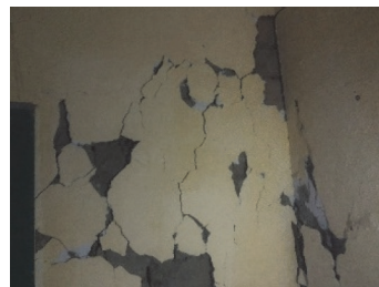
Figure 4. Earthquake damaged wall, Albania 2019
