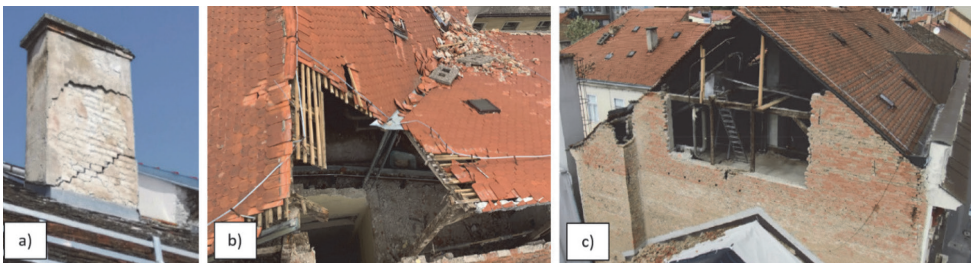
Figure 1. a) Collapse of chimneys; b) roof damage; c) collapse of attic gable wall [2]
