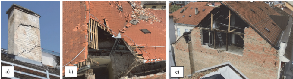
Figure 1. a) Collapse of chimneys; b) roof damage; c) collapse of attic gable wall [2]
