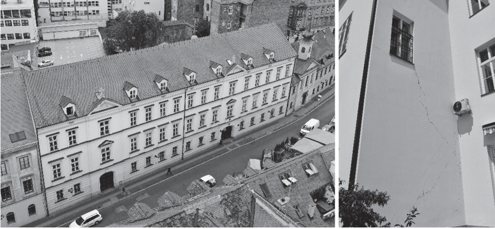
Figure 2. Educational building and damage by the earthquake
