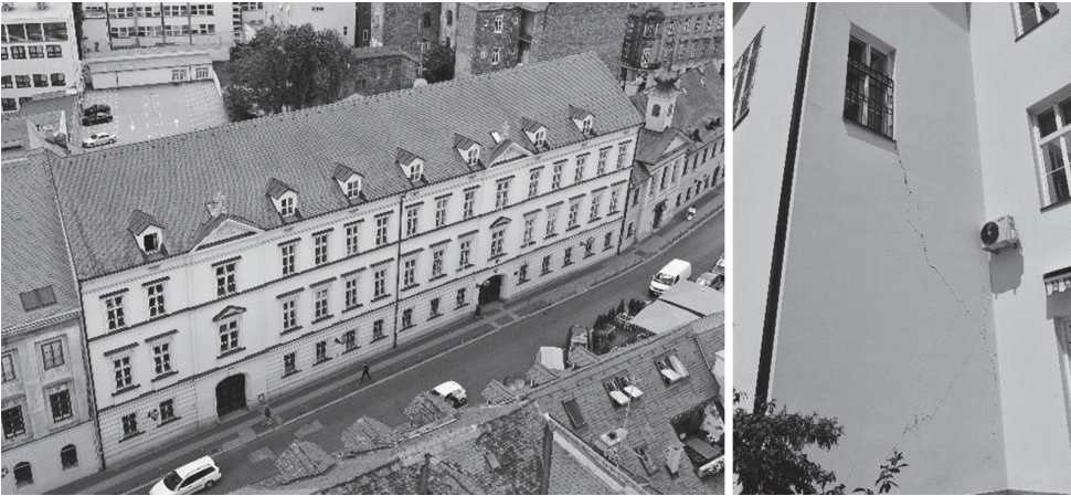
Figure 2. Educational building and damage by the earthquake
