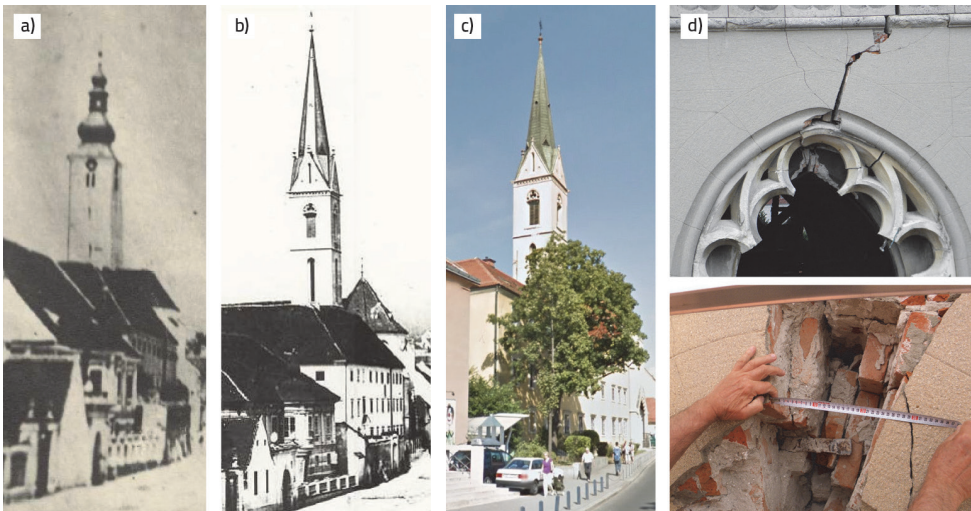
Figure 1. The bell tower of The Church of St. Francis of Assisi on Kaptol in Zagreb throughout history: a) Bell tower until 1880, b) Bell tower 1885, c) Bell tower 2020, d) Some damage of the bell tower
