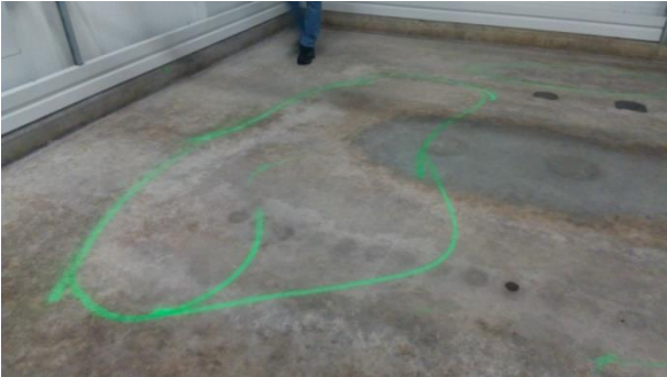
Figure 10: Surface coating spalling
