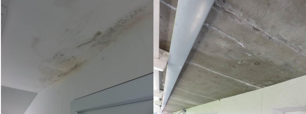
Figure 7: Leakage and lime sediments
