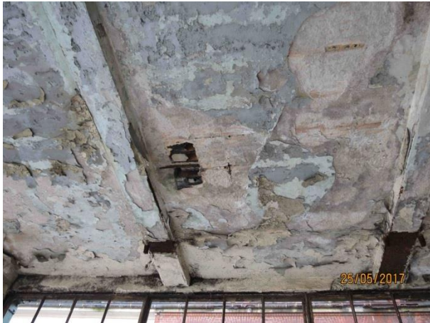
Figure 7: Destruction on Ackerman floors
