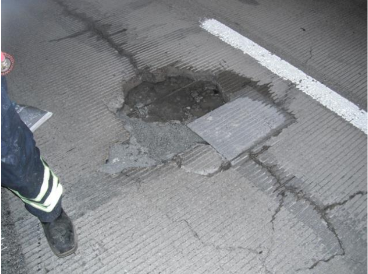
Figure 1: – Observed cracking and deterioration of the overlay requiring emergency repair procedures
