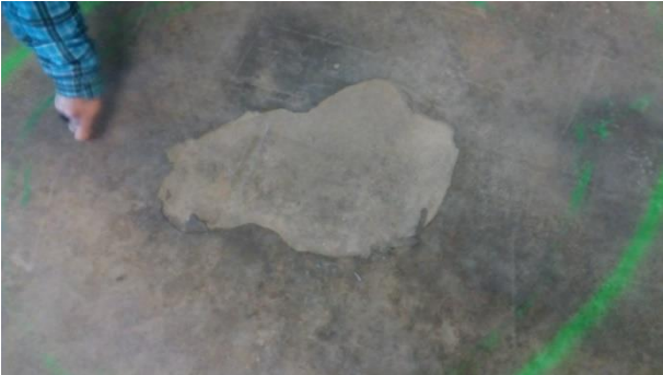
Figure 9: Surface coating spalling
