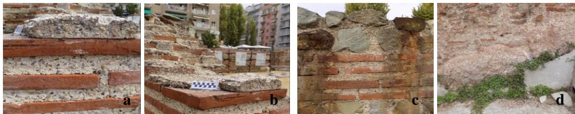
Figure 9 Deterioration phenomena of the repaired structures. a. microcracking, b. black crust, c. oxidation products, d. biological growth
