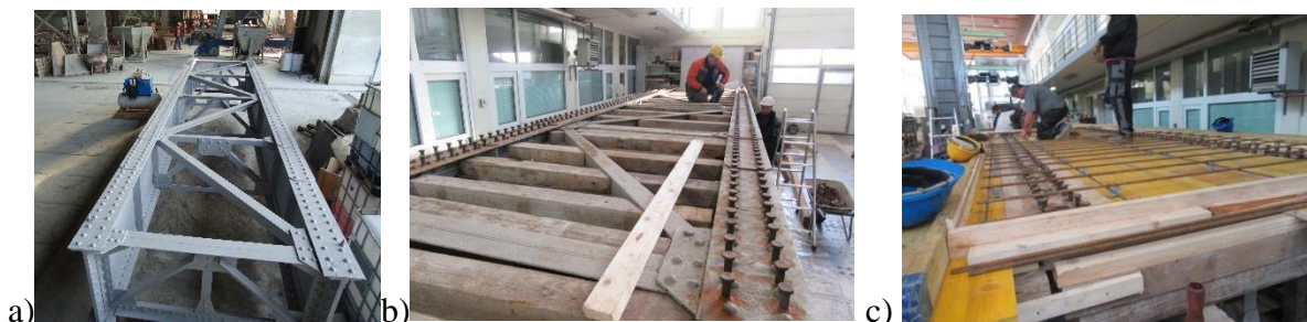
Figure 2: a) Bridge cleaned and painted, b) Welded studs, c) Secondary reinforcement and the formwork
