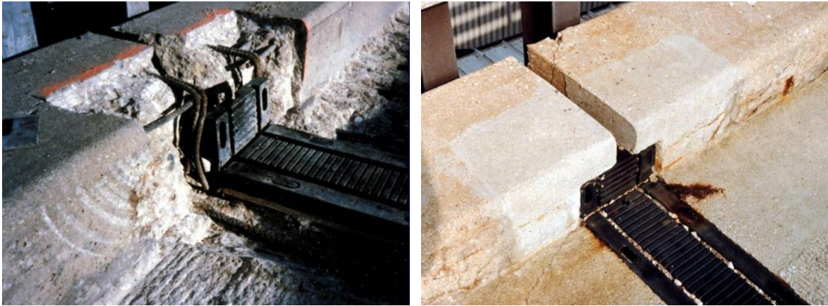
Figure 5: View of patches performed at Argonne bridge. Surface preparation of the concrete to the left, and condition of those repairs 10 years after to the right
