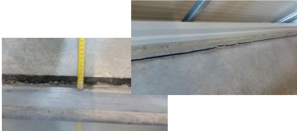
Figure 11: Joint gap at slab-beam connection
