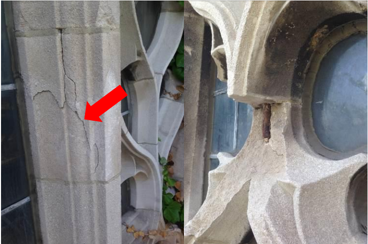
Figure 2 - Cracked and spalled window mullions and rosettes
