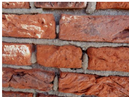
Figure 4: Damage in a trass-lime repointing caused by incomplete hydration of the binding system.
