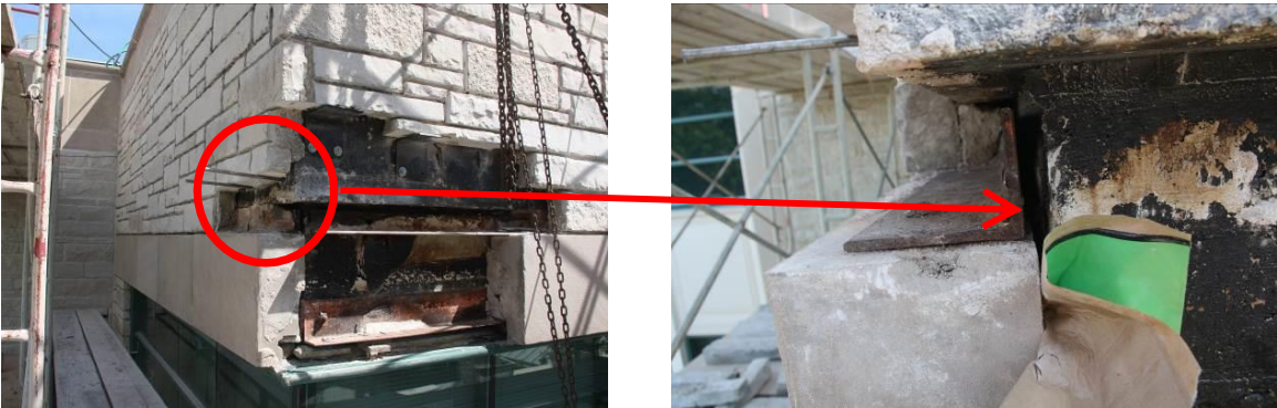
Figure 4 - Overall and close up view of shelf angle detached from structural beam and cracked limestone panel at the back side due to corrosion of shelf angle
