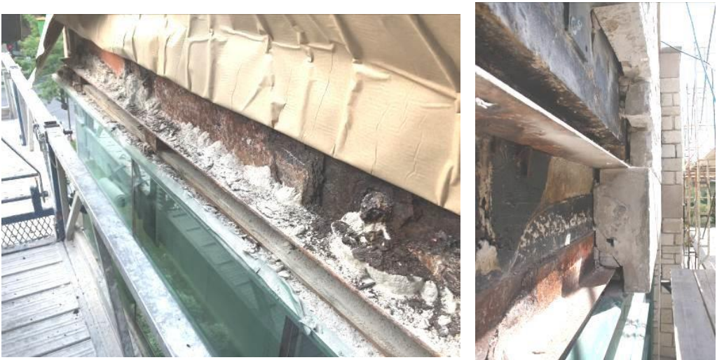
Figure 3 - Severely corroded steel shelf angle and cracked and spalled limestone block due to corrosion
