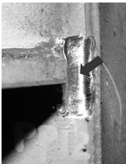
Figure 11: Highlighted fatigue crack in web gap using MT method
