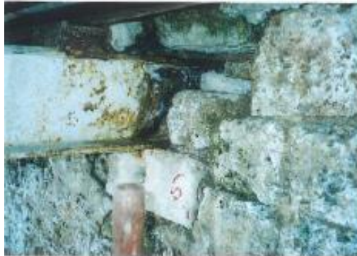
Figure 3: Corrosion of the steel and carbonization of stone [13]
