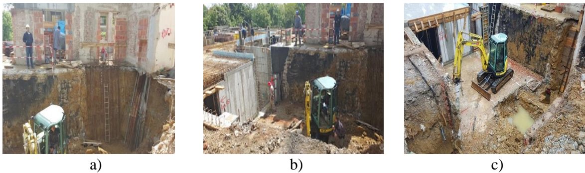
Figure 1: a) cleaning the old walls for preparation for building of the new walls on joints with the old ones b) a newly built basement and a junction with the old wall of the house, c) excavating of the elevators pit
