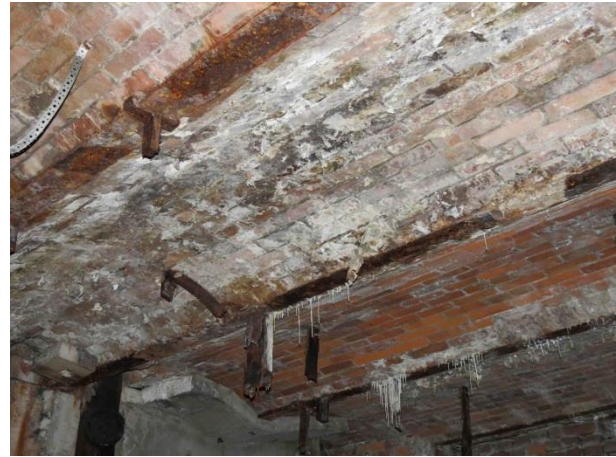
Figure 12: Destruction of brick masonry floors
