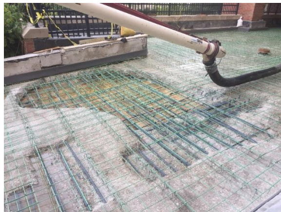
Figure 2: Surface preparation of concrete and coating of reinforcing bars at partial and full depth patches, and installation of new epoxy coated bars for bonded overlay
