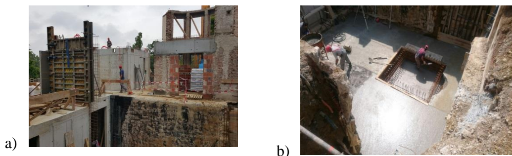
Figure 2: a)work in progress, new walls are being built, b) the floor concrete slab and the foundation of the elevator pit are performing
