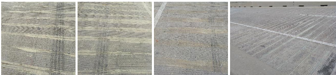
Figure 9: Area repaired after 6 months of traffic. On the two pictures on the left one of the large longitudinal cracks along the beam can be observed being crossed by the FRP strips. No further deterioration was observed since the installation of the NSM FRP strips.
