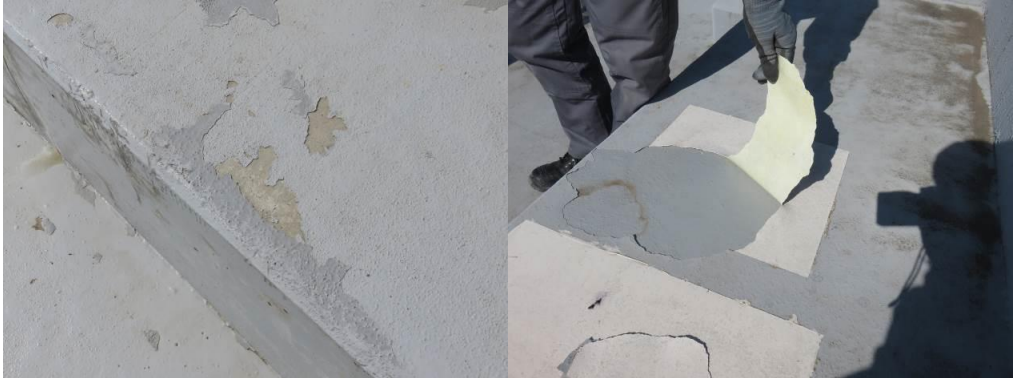
Figure 5: Surface coating deterioration (spalling, peeling...)
