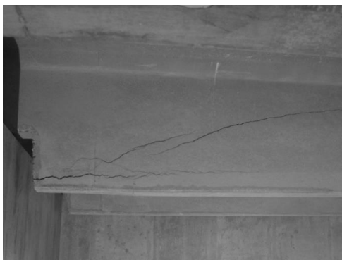
Figure 1: Diagonal shear cracking and longitudinal cracking in stem
