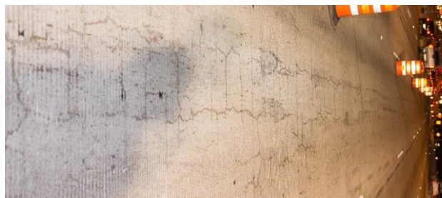
Figure 4: Cracking pattern in one of the East-bound lanes
