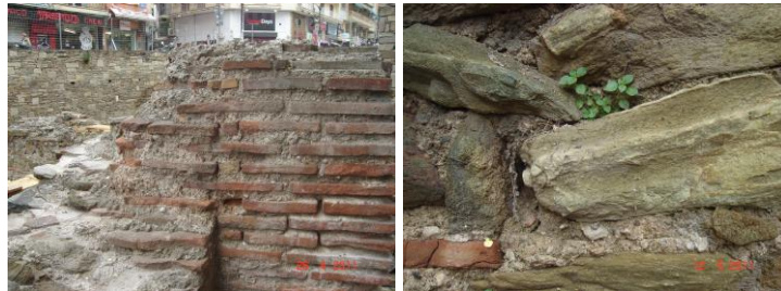
Figures 5-6 Deterioration problems of the masonries before the intervention works.
