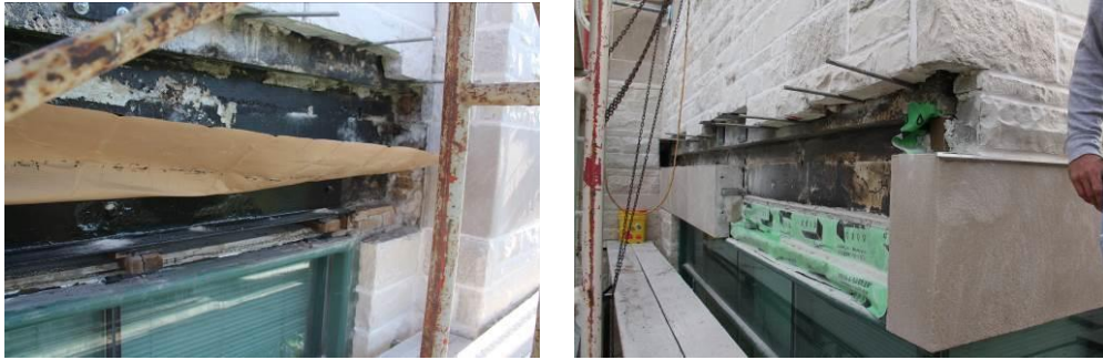
Figure 9 - Repair 6, repairing of steel shelf angles / window lintels at building built in
