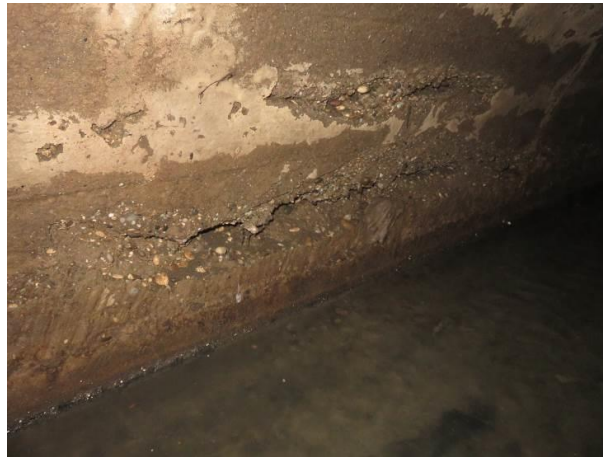
Figure 4: Deterioration of the concrete cladding
