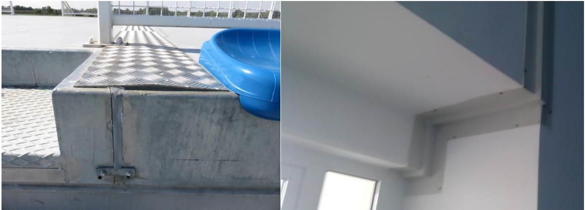
Figure 4: Unsatisfactory crack repair (upper and lower side of the structure)
