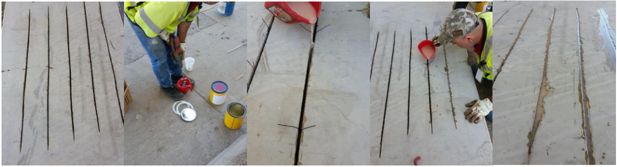
Figure 7: Test installation – from left to right: saw cuts, mixing of epoxy resin, FRP strip introduced and maintained in place using wires, filling of the slot with epoxy resin and result
