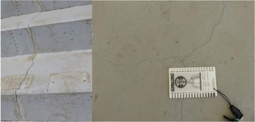
Figure 6: Typical cracks in upper surface
