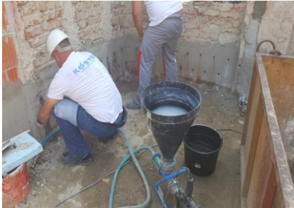
Figure 5: injection into the zone of contact with the ground (STABILCEM, MAPESTOP, LAMPOCEM, MAPE-ANTIQUE INTONACO NHL)
