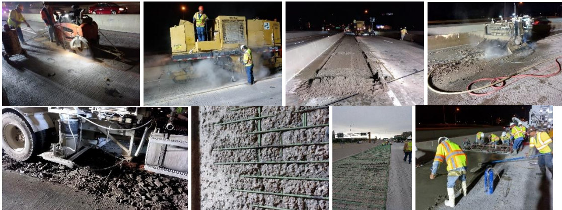
Figure 6: Demolition and reconstruction of overlay – from left to right, top to bottom: Saw cutting of demolition perimeter, milling machine, result of milling, hydrodemolition machine, aspirator truck helping clear debris, left-over rough surface showing original slab, new reinforcement mat in place, and concreting.
