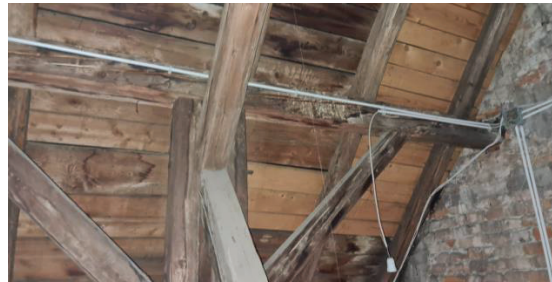
Figure 9: Failure of timber elements due to water leakage and seismic excitations (photo credit: Studio Arhing d.o.o.)
