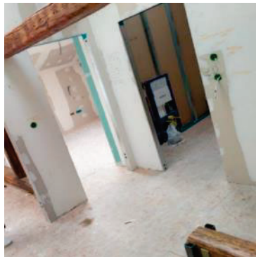
Figure 11: Improper attic modifications (photo credit: HCPI [4])
