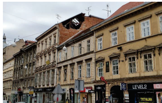
Figure 4: Failure of gable walls (photo credit: M. Stepinac)
