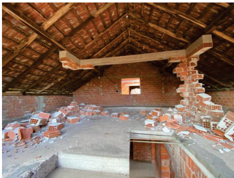
Figure 12: Improper attic modifications (photo credit: HCPI [4])
