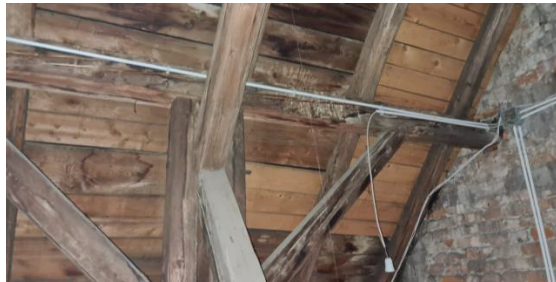
Figure 9: Failure of timber elements due to water leakage and seismic excitations (photo credit: Studio Arhing d.o.o.)
