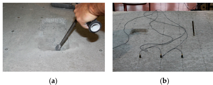
Figure 4. Discrete damages on the RC plate: (a) chiseling; (b) one of the damage locations on the concrete plate.
