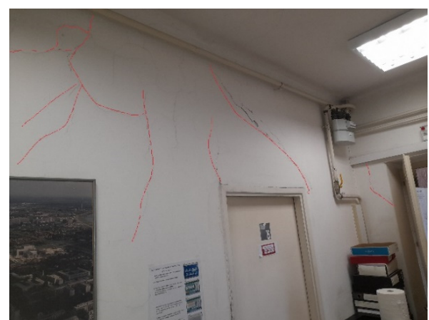
(b) First floor damage
