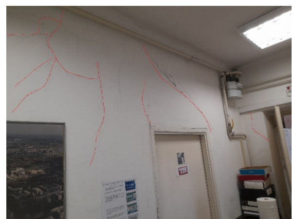
(b) First floor damage
