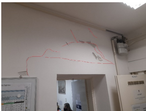
(a) Ground floor damage
