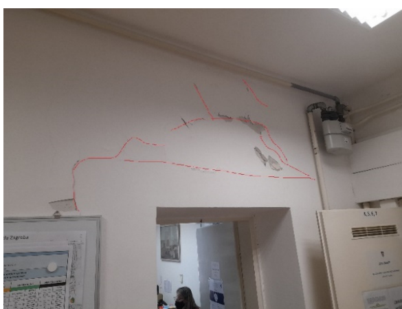
(a) Ground floor damage
