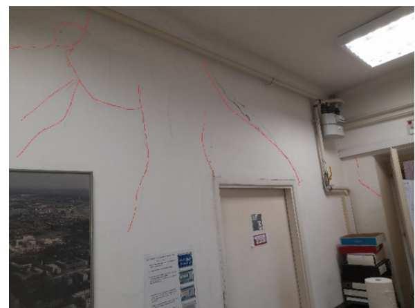
(b) First floor damage
