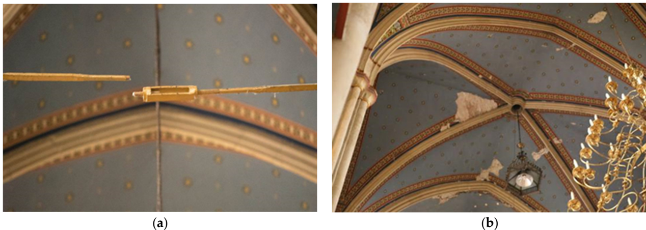
Figure 1. Cathedral of the Assumption of Mary, Zagreb: (a) Fractured tie rod after its load bearing capacity was reached (b) Damaged vaults after the March 22nd 2020 Zagreb earthquake.
