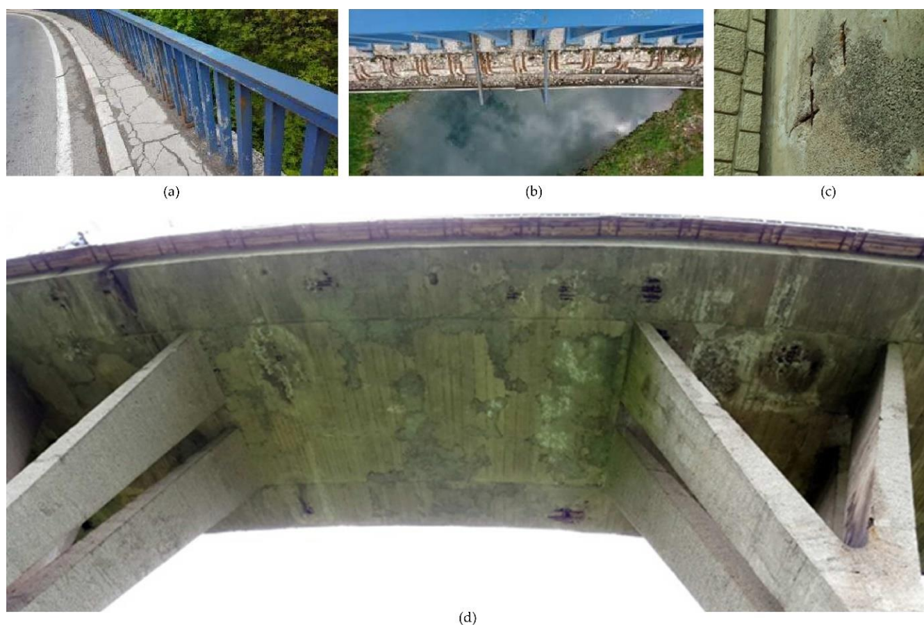
Figure 5. Most significant damages to Rastoke Bridge [48]: (a) degradation of corrosion protection coating of the pedestrian fence due to poor protection and lack of maintenance; (b) breakage of the concrete cover and reinforcing steel corrosion of the cornice due to freezing and thawing; (c) segregation due to poor concreting and reinforcing steel corrosion leading to a concrete spalling at the bottom slab next to the abutment; (d) delamination of the concrete cover and efflorescence at the bottom of the slab due to wetting and probable damage in waterproofing. Reprinted with permission from ref. [48]. 2019. IABSE.
