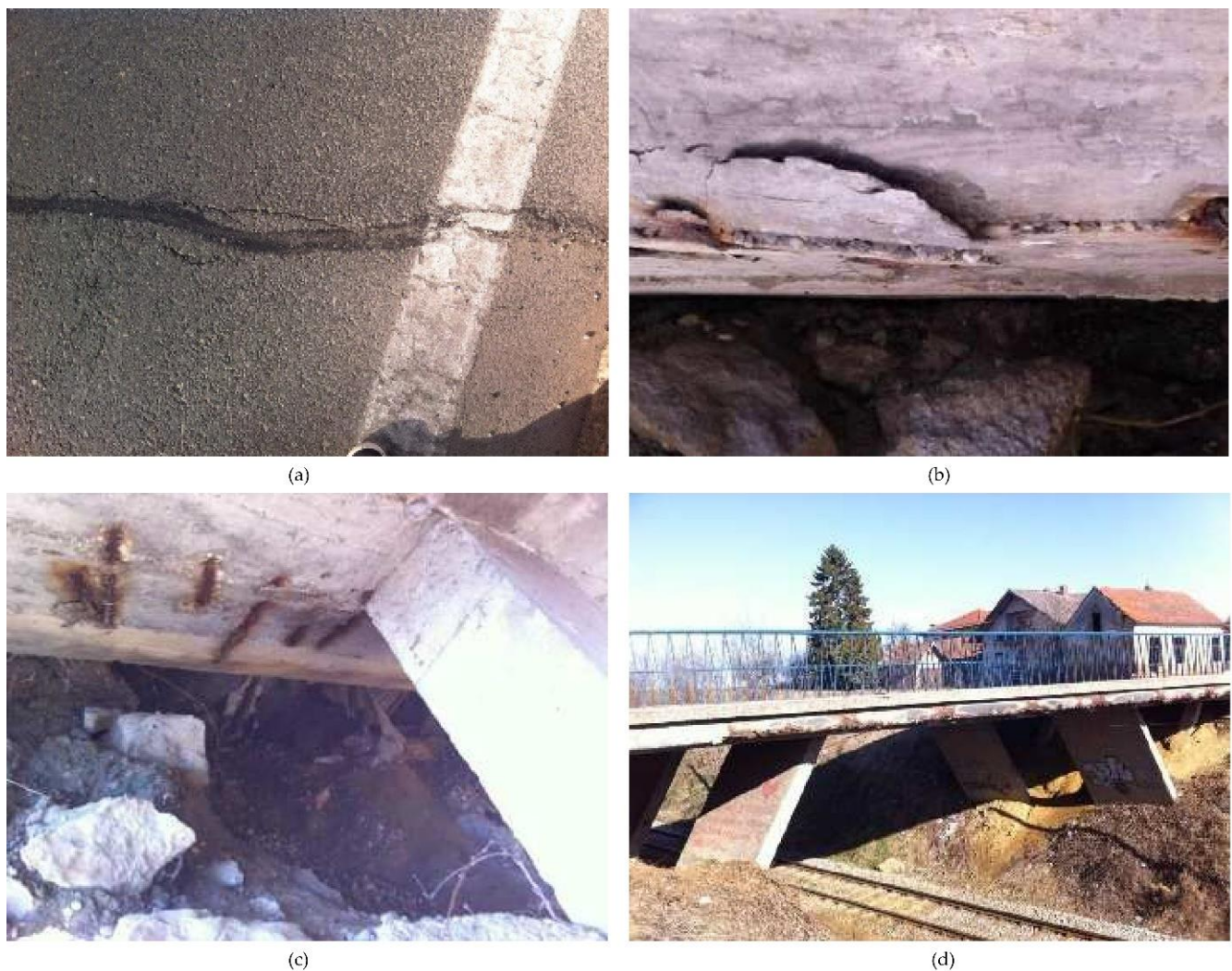
Figure 6. Most significant damages to Bjelovar Bridge [48]: (a) repaired cracks in asphalt pavement on the transfer location from the bridge to the approach road; (b) concrete cover fraction and (c) reinforcement steel corrosion on the underside of the superstructure slab near the junction with the side legs of the V-shaped piers; (d) soil erosion at the embankment cone. Reprinted with permission from ref. [48]. 2019. IABSE.
