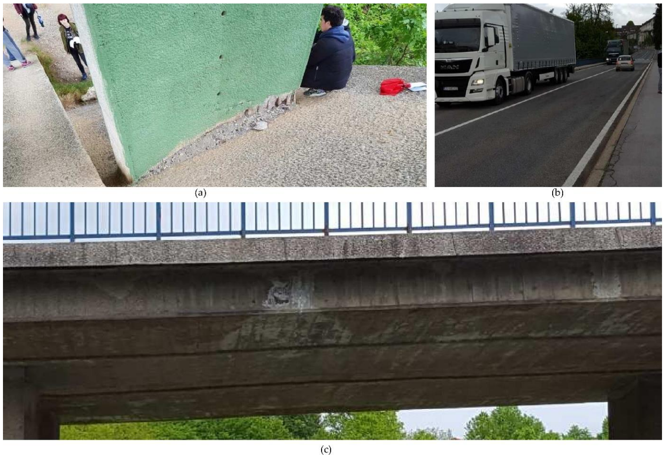
Figure 4. Most significant damages to Slunjčica Bridge [48]: (a) concrete cover fraction and reinforcing steel corrosion at the pier due to the insufficient concrete cover and poor construction; (b) sidewalk block cracking probably due to vibration and poor construction concrete; (c) cover fraction and reinforcing steel corrosion at the slab bottom due to insufficient concrete cover and efflorescence appearance due to wetting and probable damage in waterproofing. Reprinted with permission from ref. [48]. 2019. IABSE.
