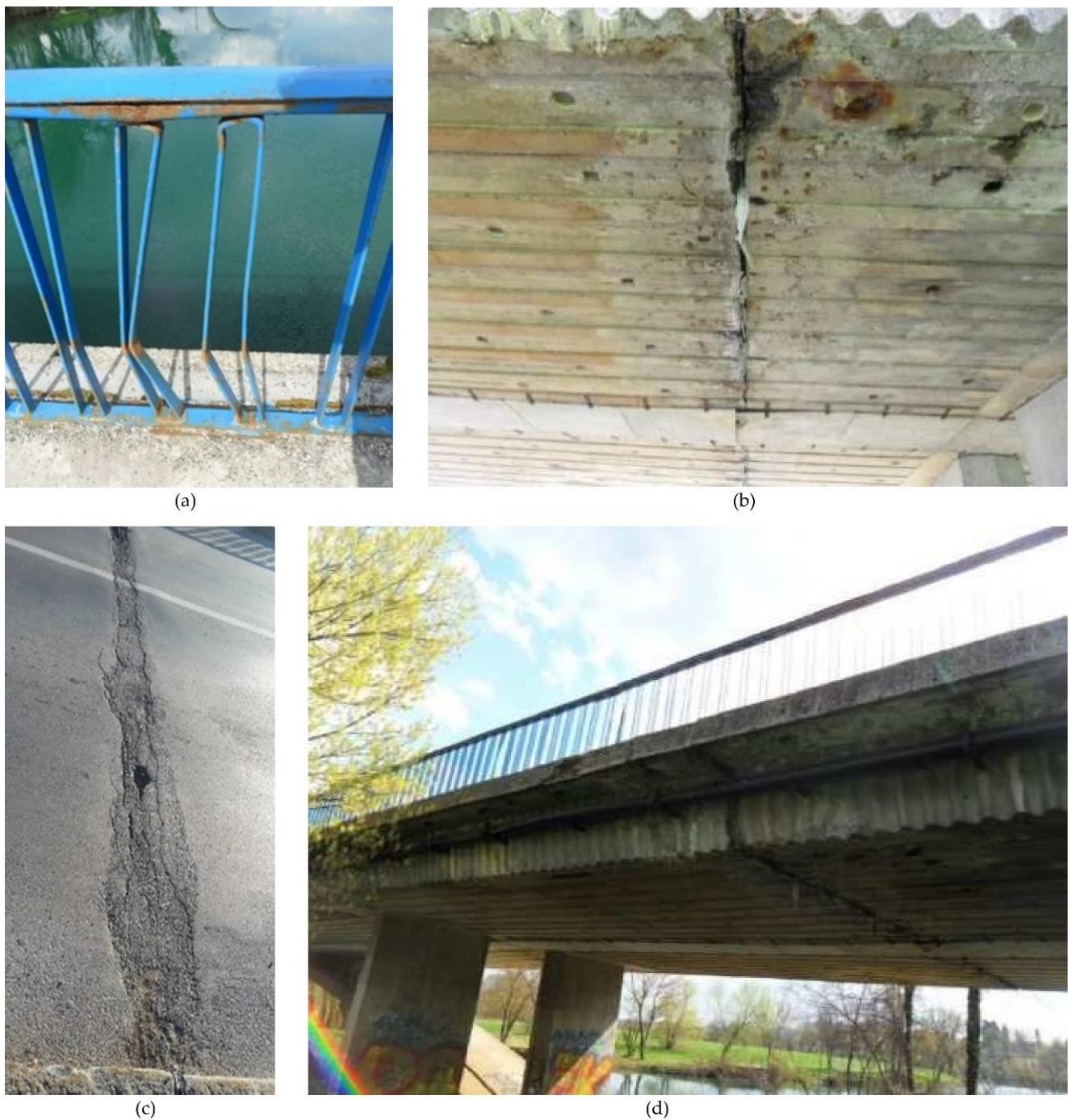
Figure 7. Most significant damages to Korana Bridge [48]: (a) mechanical damage and corrosion of the pedestrian fence due to poor protection and lack of maintenance; (b) construction joint, concrete wetting, and efflorescence on the main slab girders below (c); (c) cracks in the asphalt pavement and dilatation in connections with the construction joint in the 8th field of the superstructure deck close to the pier; (d) cornice delamination. Reprinted with permission from ref. [48]. 2019. IABSE.
