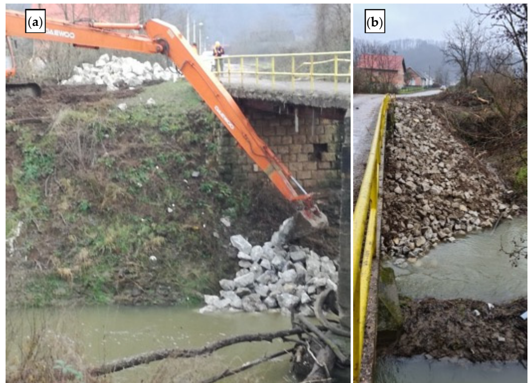
Figure 15. Immediate measures to secure the abutment of Matija Gubec street bridge: (a) beginning of the work; (b) completed infill.
