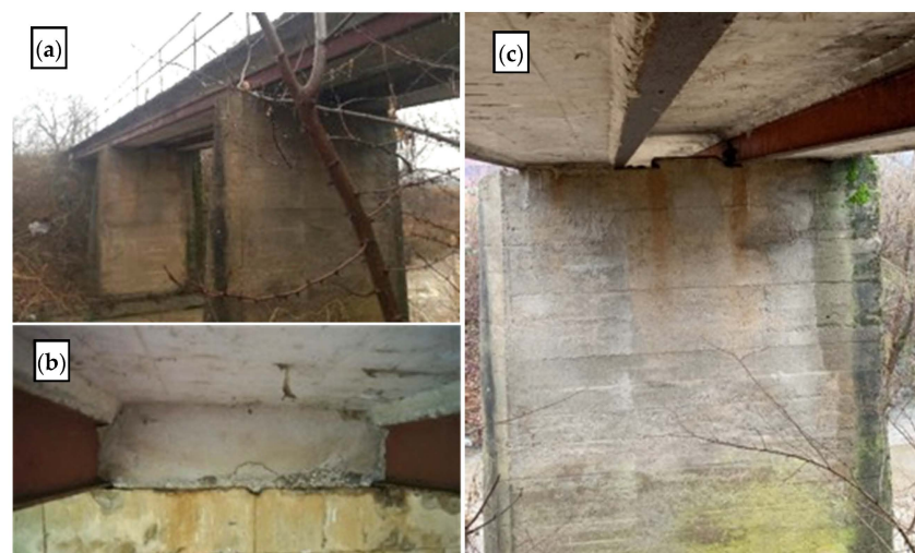
Figure 12. Nikola Tesla street bridge: (a) view of the bridge; (b) main girders to abutment support; (c) superstructure under view.
