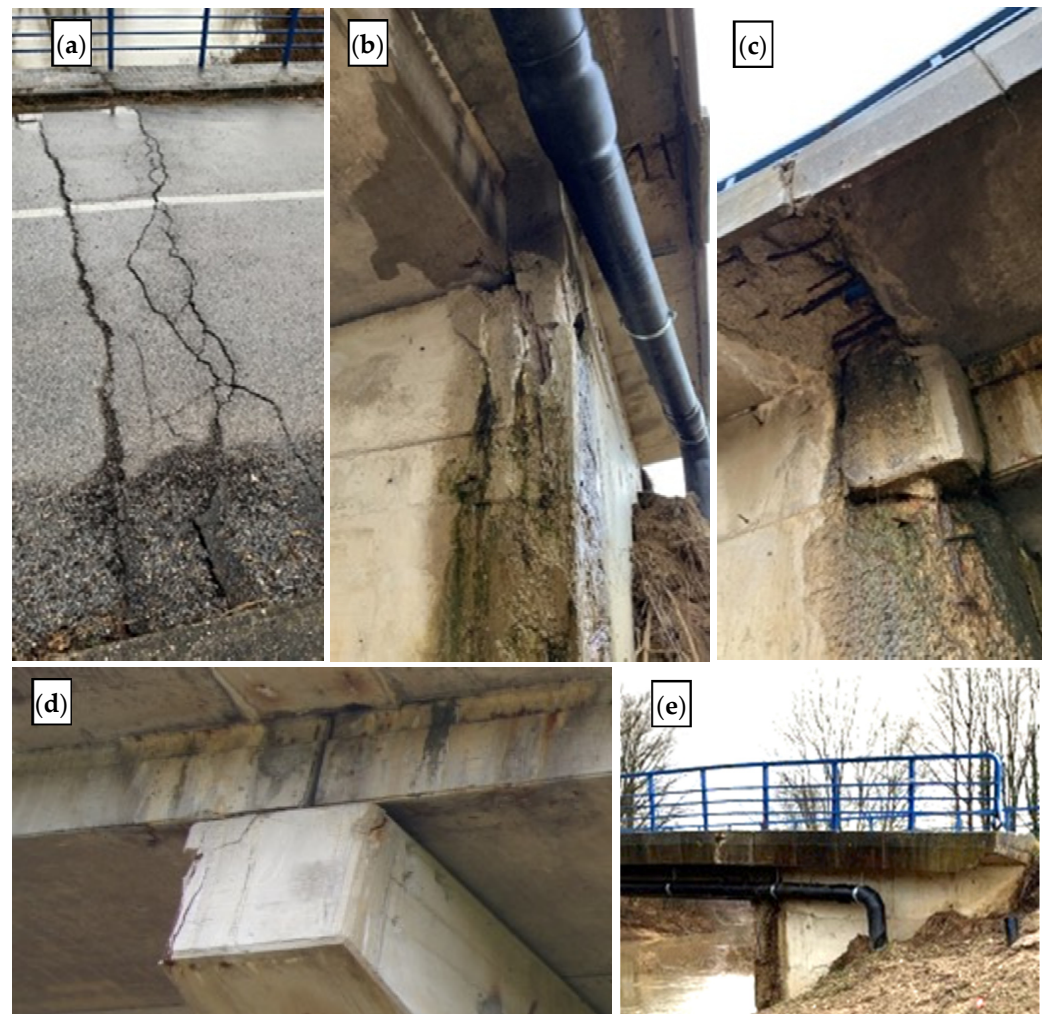
Figure 14. Hađer bridge: (a) damage caused by earthquake in the asphalt; (b) fractured abutment side wall due to the earthquake; (c) water leakage from superstructure end, causing damage to abutment; (d) uneven support length for the girders; (e) cracked cornice due to earthquake movement.
