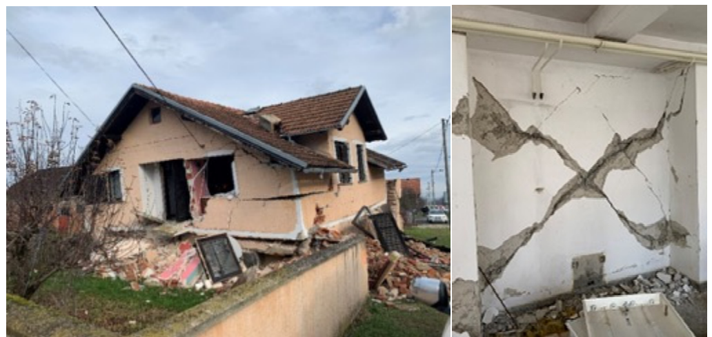
Figure 1. DG4 and DG5 damage from the December 2020 earthquake in Sisak-Moslavina county.
