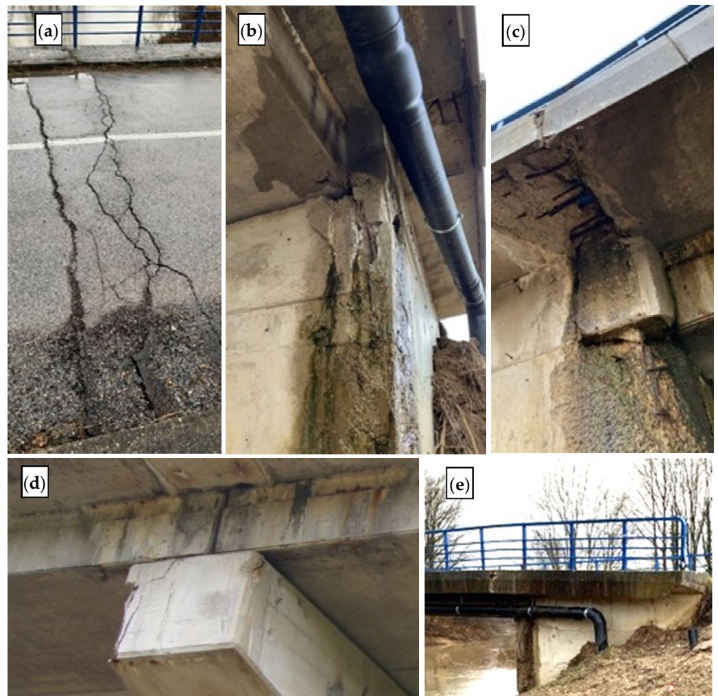
Figure 14. Hađer bridge: (a) damage caused by earthquake in the asphalt; (b) fractured abutment side wall due to the earthquake; (c) water leakage from superstructure end, causing damage to abutment; (d) uneven support length for the girders; (e) cracked cornice due to earthquake movement.
