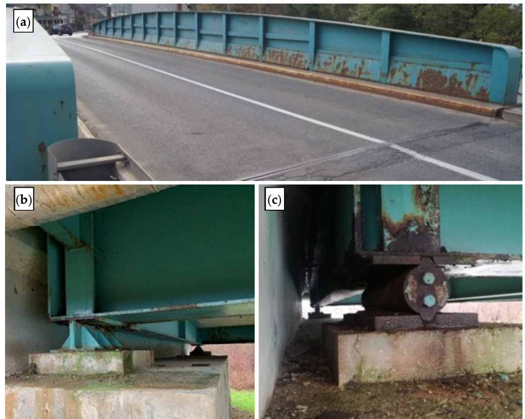
Figure 7. Glina bridge: (a) main girder and carriageway; (b) fixed bearing; (c) movable bearing.
