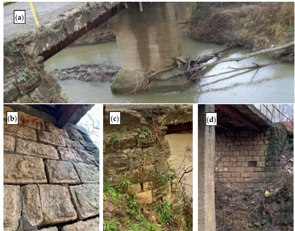
Figure 8. Matija Gubec street bridge: (a) columns—large foundation for the column in the middle of the riverbed and scour visible on the east column; (b) abutment stone wall damage; (c) abutment sliding signs; (d) evidence of subsequent abutment sliding—stone wall integrity compromised.
