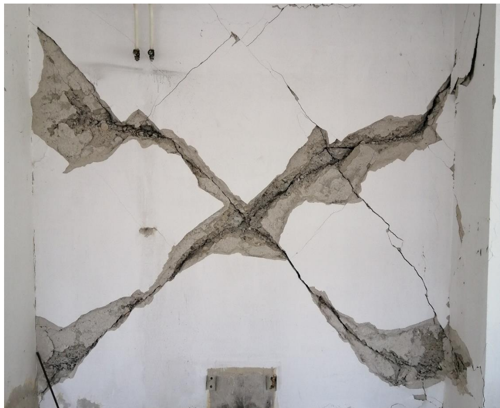
Figure 2. Diagonal cracks in the lightly reinforced RC shear wall.
