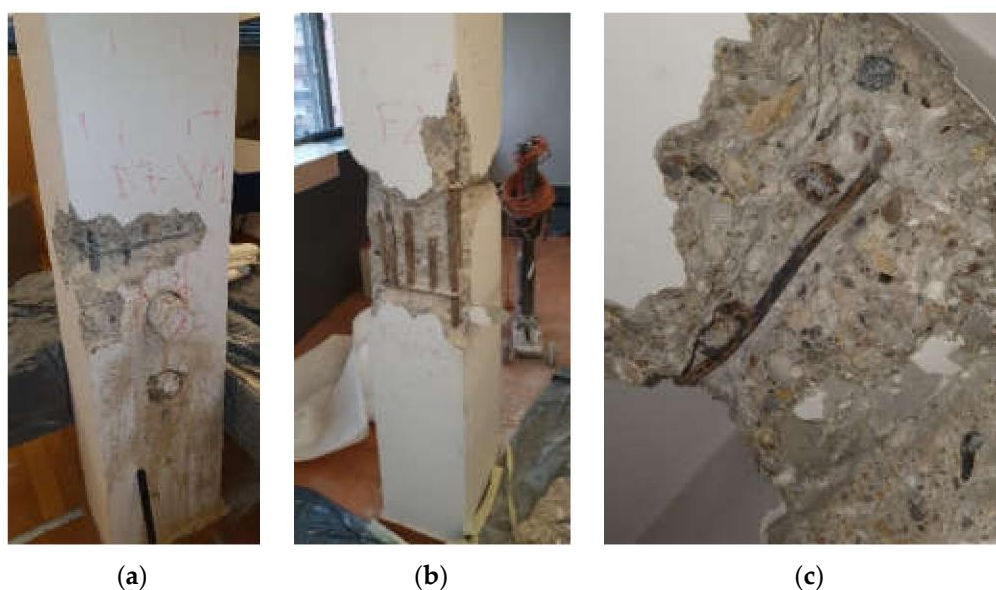
Figure 13. Column on the ground floor (a), second floor (b), and a beam on the 2nd floor (c).
