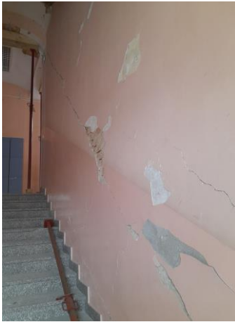
In-plane shear failure of interior walls
