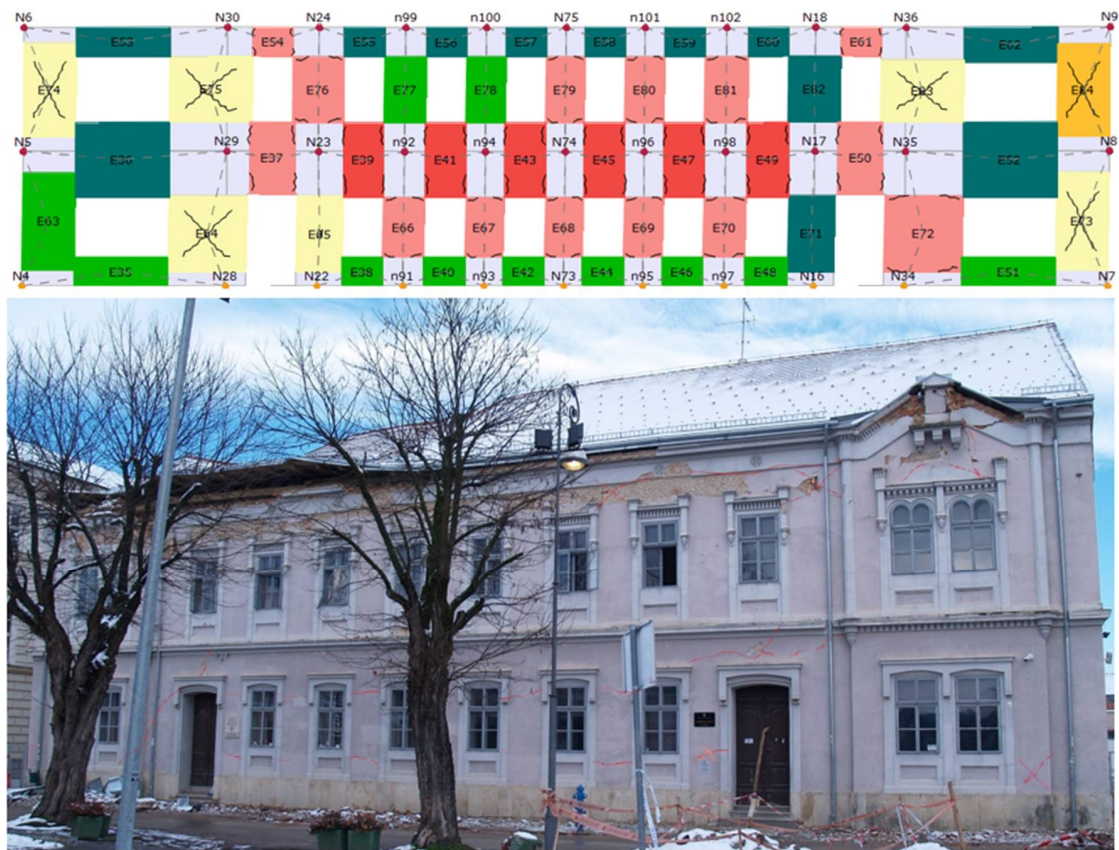
Figure 16. Detailed display of street facade damage in the 3Muri software package and actual damage to the street facade of the building in question.
