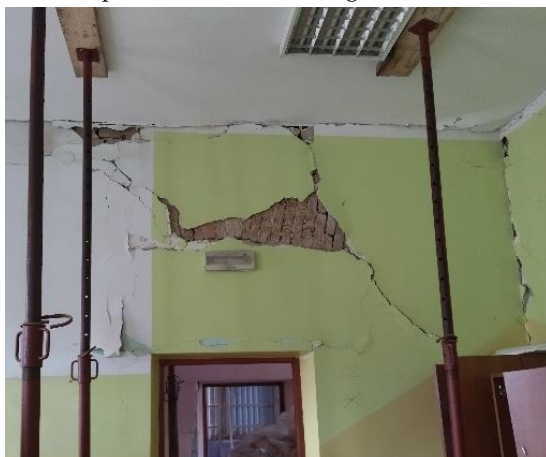
Shear failure of spandrels (diagonal cracks)
