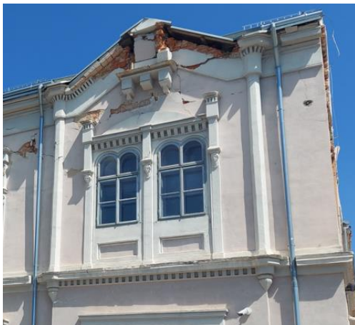
Out-of-plane wall failure in the attic
