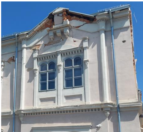
Out-of-plane wall failure in the attic
