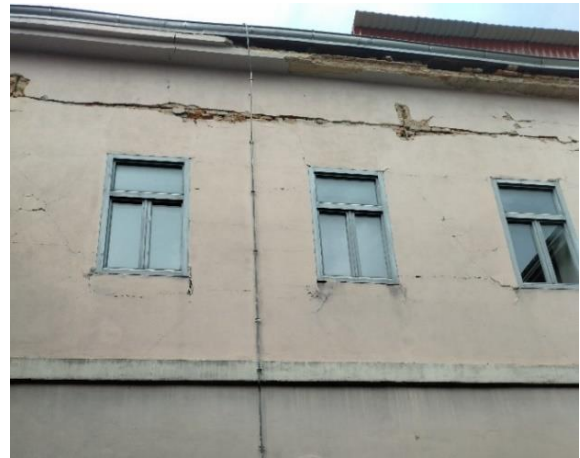
In-plane sliding failure (horizontal cracks)
