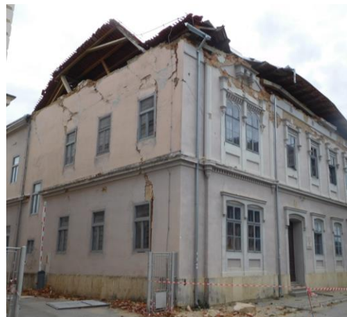
Partial overturning of the gable walls
