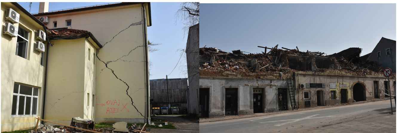
Figure 2. Damaged buildings in the historical center of Petrinja.
