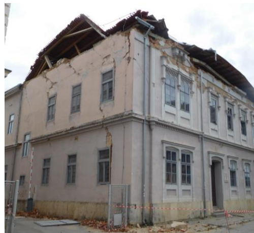
Partial overturning of the gable walls
