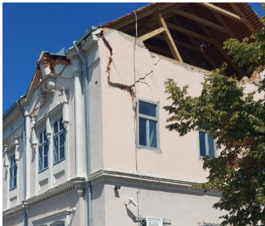
Out-of-plane failure of wall connections
