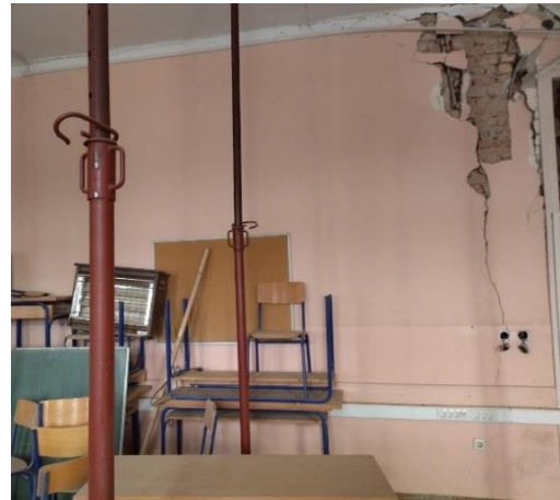
Tensile failure of masonry and vertical cracks at the corners
