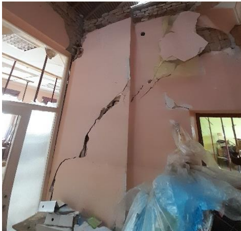
In-plane shear failure (diagonal cracks)
