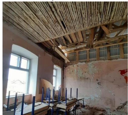
Partial collapse of the floor structure
