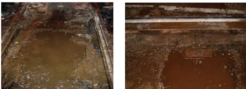
Figure 3. Condition of the closed track formation during the most part of year
