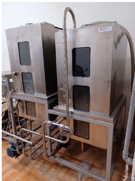
Figure 1. Pilot plant for the treatment of oily wastewater using pretreatment and EF/EC processes.
