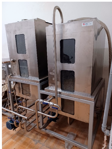
Figure 1. Pilot plant for the treatment of oily wastewater using pretreatment and EF/EC processes.
