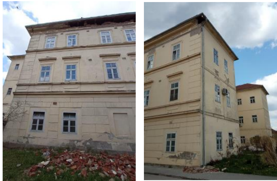
Figure 10. Damage to the facade.
