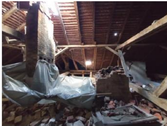
Figure 11. Collapsed chimney and damaged roof covering.
