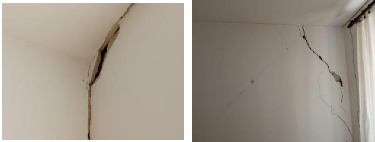
Figure 9. Cracks at the junctions of load-bearing walls.
